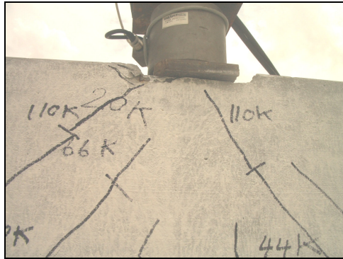
Figure C.21 At 110 kips, some cracks became longer to reach position of load point
