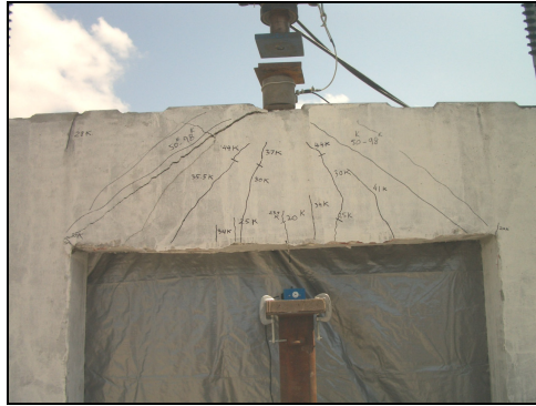
Figure C.10 The wall lost all of stiffness at load 98 kips
