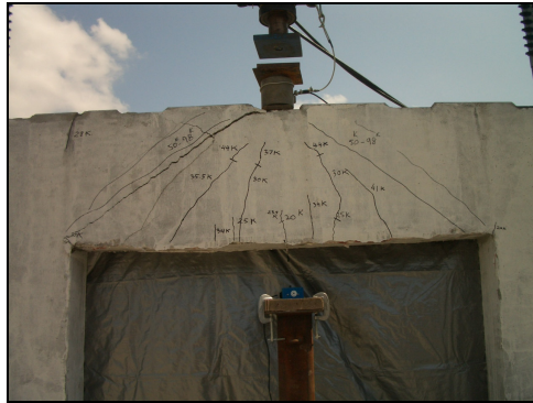
Figure 3.16 Wall panel with window opening after test
