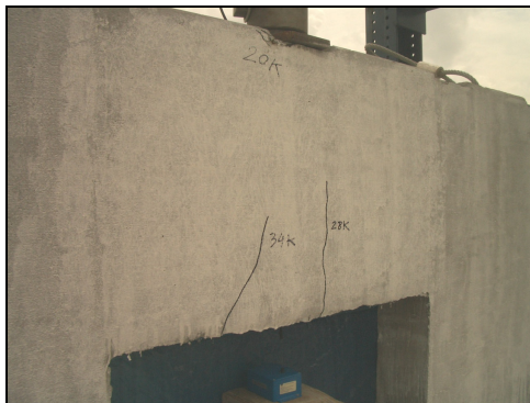
Figure C.15 Find another flexural crack at the left of the first crack at 34 kips
