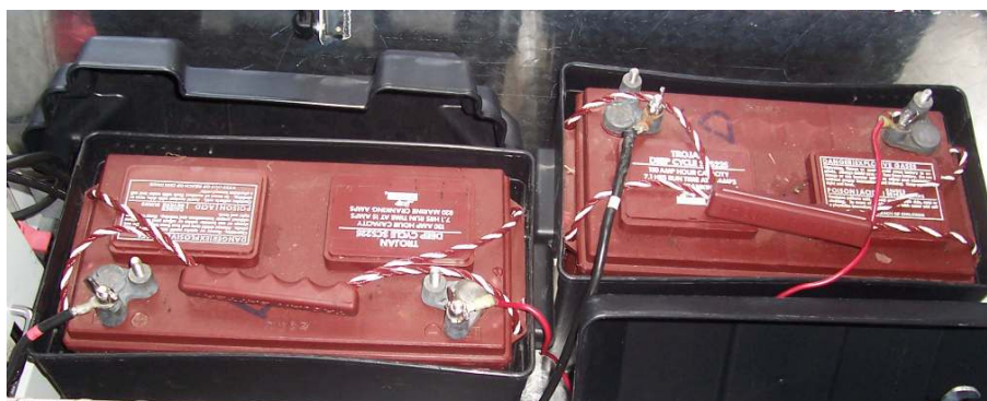
Figure 3.10 12 - Volt deep cycle batteries
