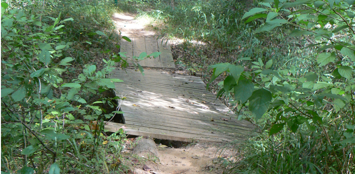
Fig. 4.108 Bridge that needs repair
