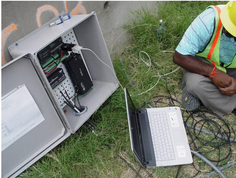
Figure 6.6 CR10X Data logger and on site data transfer to LAPTOP
