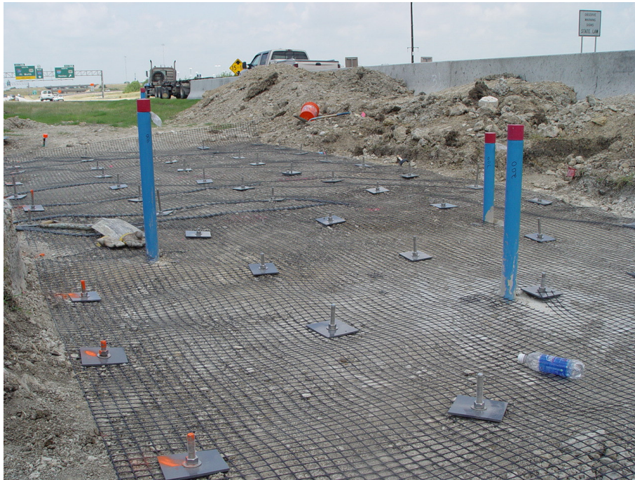
Figure 5.21 Test section after fastening geogrid to DSM columns using anchor rod and plate-bolt system.
