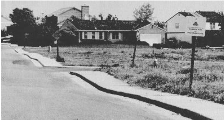
Figure 2.3 Pavement overlying expansive subsoils and subjected to distress due swell-shrink movements (source: www.surevoid.com )
