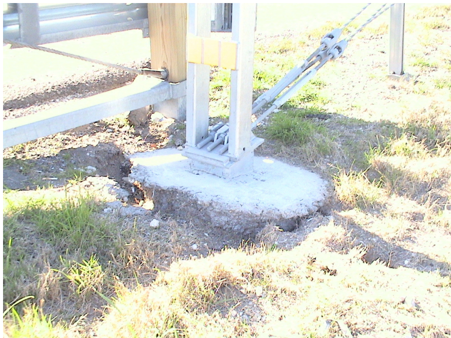
Figure A.25 Foundation Failures of 3-cable Median Barriers Built on Expansive Soils at US 80 Eastbound Sta. 110+96
