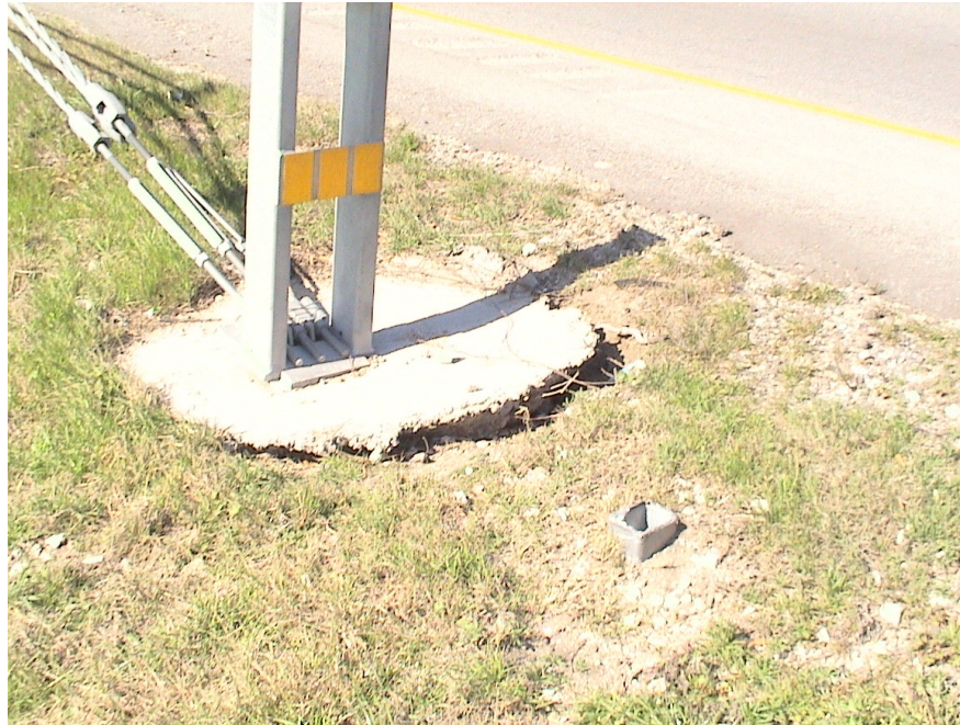
Figure A.26 Foundation Failures of 3-cable Median Barriers Built on Expansive Soils at US 80 Westbound Sta. 111+27
