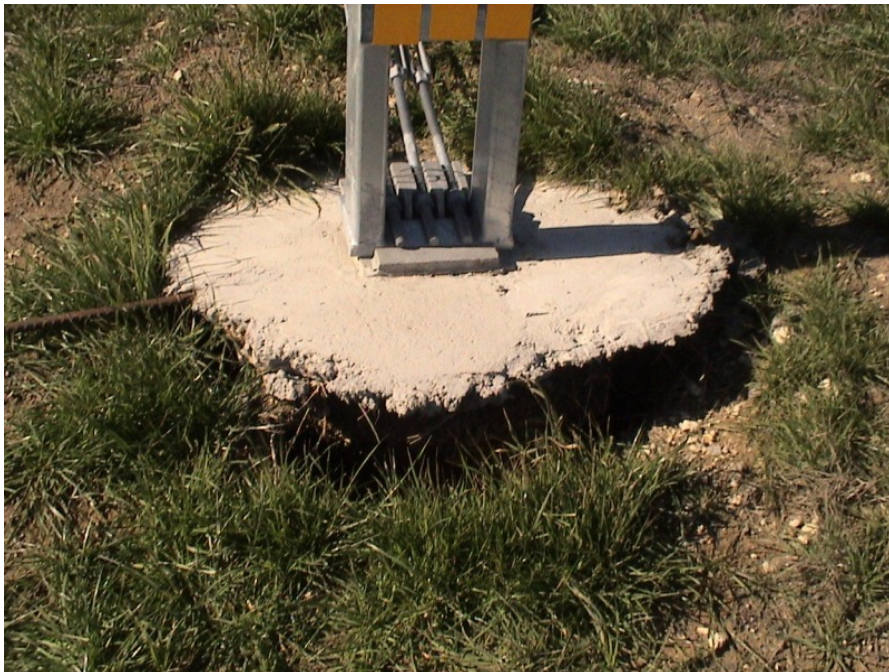
Figure A.6 Foundation Failures of 3-cable Median Barriers Built on Expansive Soils at IH 20 Westbound Sta. 862+19
