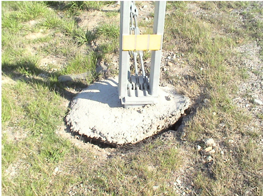
Figure A.23 Foundation Failures of 3-cable Median Barriers Built on Expansive Soils at US 80 Eastbound Sta. 81+50
