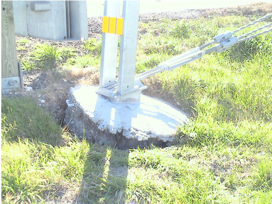
Figure A.21 Foundation Failures of 3-cable Median Barriers Built on Expansive Soils at US 80 Eastbound Sta. 77+37
