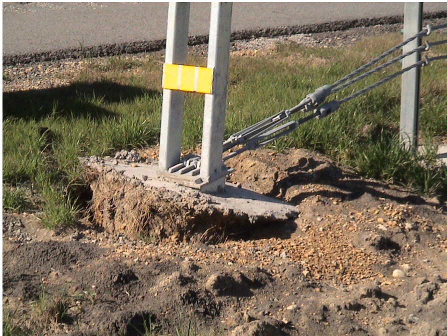
Figure A.12 Foundation Failures of 3-cable Median Barriers Built on Expansive Soils at US 175 Eastbound Sta. 149+98
