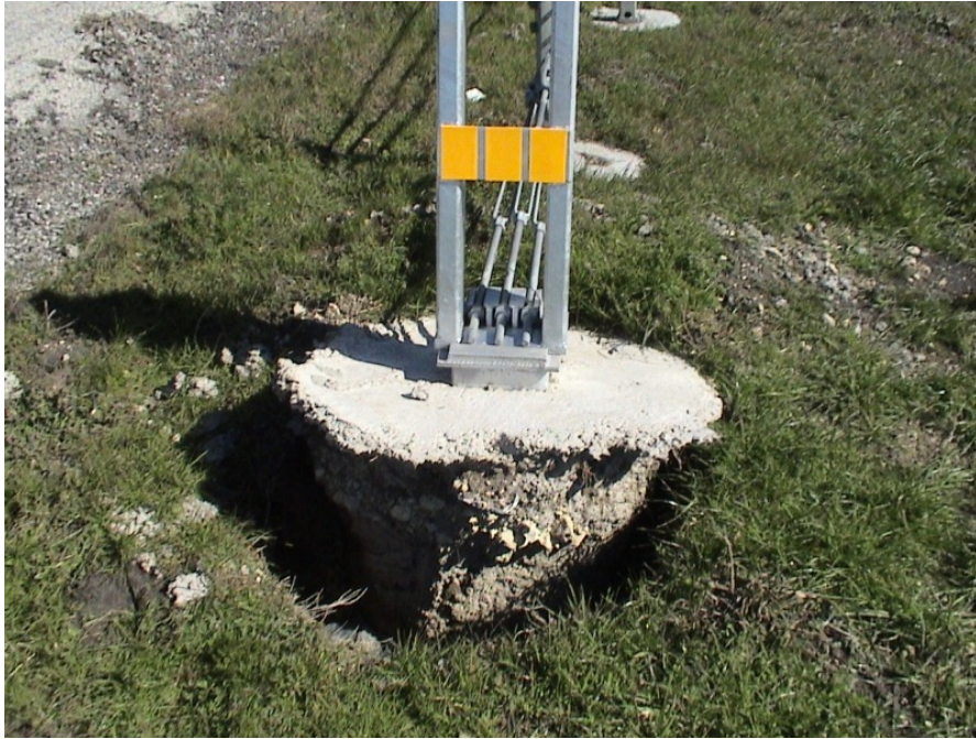
Figure A.5 Foundation Failures of 3-cable Median Barriers Built on Expansive Soils at IH 20 Westbound Sta. 973+44
