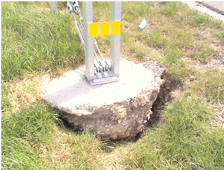
Figure A.31 Foundation Failures of 3-cable Median Barriers Built on Expansive Soils at US 80 Eastbound Sta. 438+28
