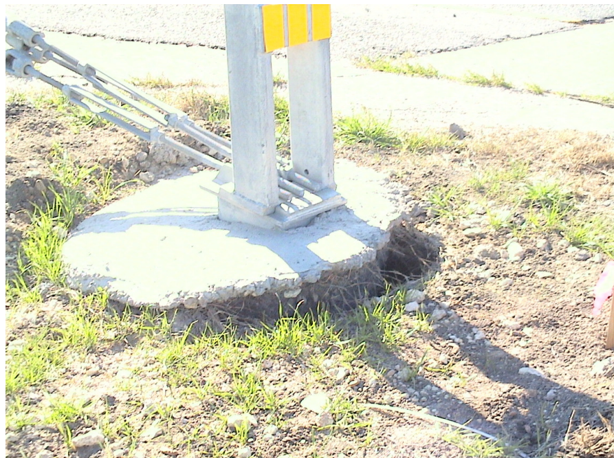
Figure A.14 Foundation Failures of 3-cable Median Barriers Built on Expansive Soils at US 175 Eastbound Sta. 92+00
