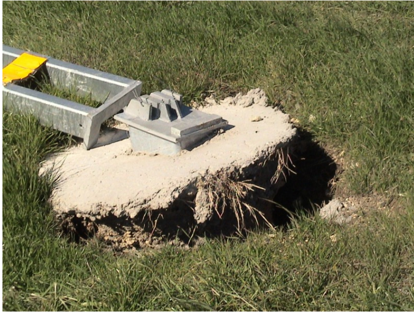
Figure 2.3 Foundation Failures of 3-cable Median Barriers Built on Expansive Soils at IH 20 Westbound Sta. 1069+00
