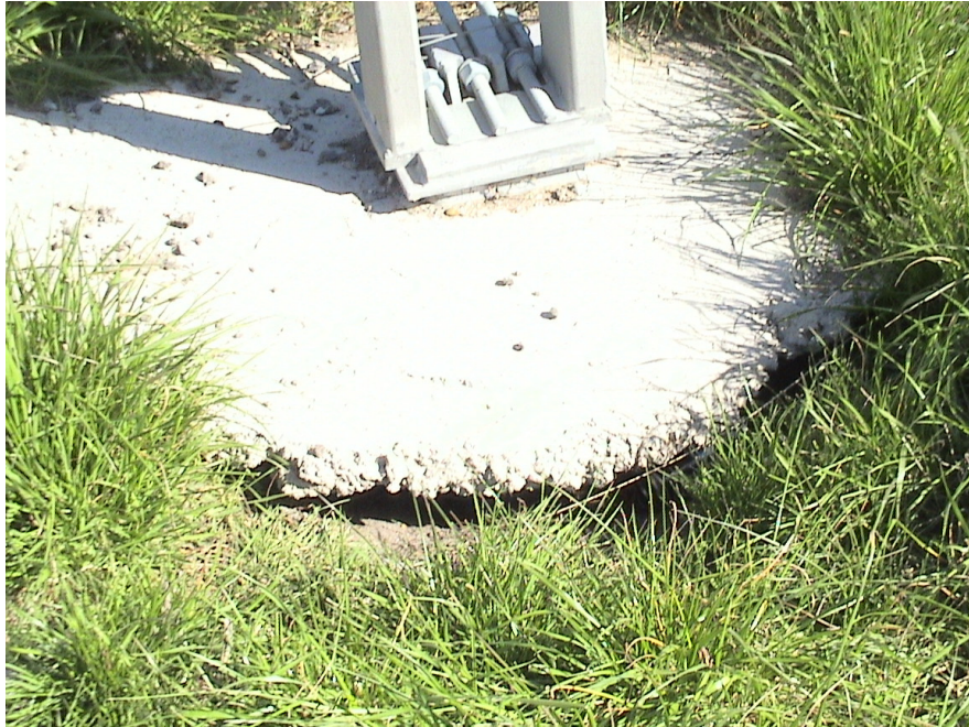
Figure A.20 Foundation Failures of 3-cable Median Barriers Built on Expansive Soils at US 80 Westbound Sta. 65+21
