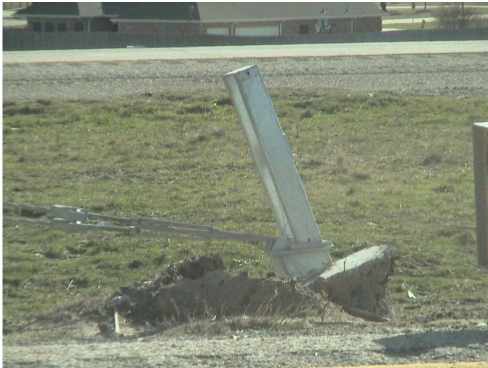
Figure A.10 Foundation Failures of 3-cable Median Barriers Built on Expansive Soils at IH 20 Westbound Sta. 903+00
