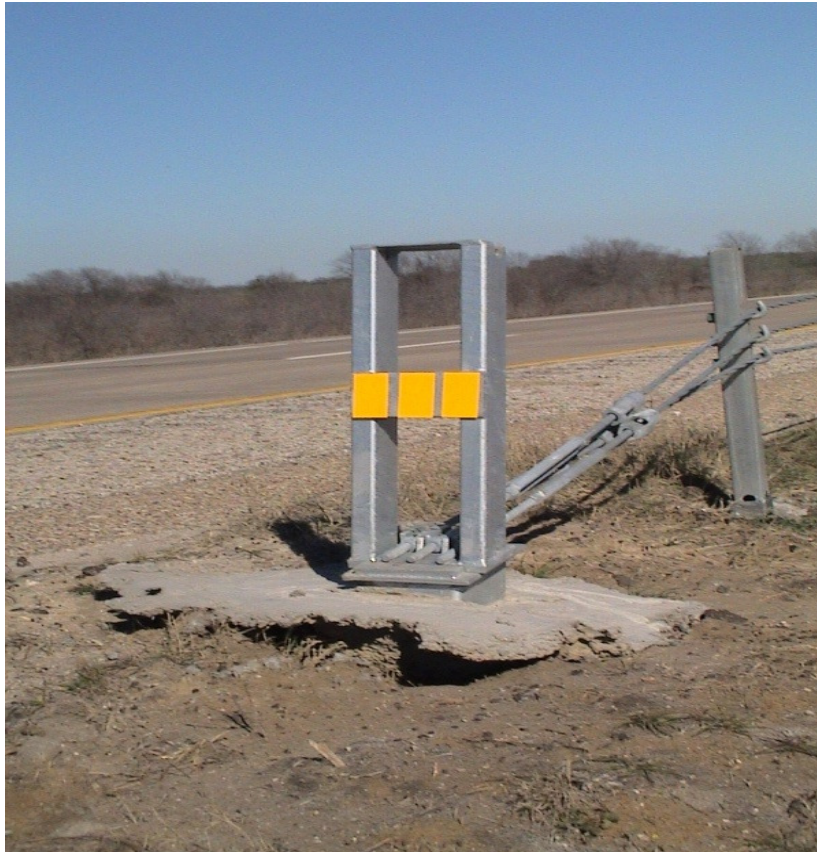
Figure A.9 Foundation Failures of 3-cable Median Barriers Built on Expansive Soils at IH 20 Westbound Sta. 976+27
