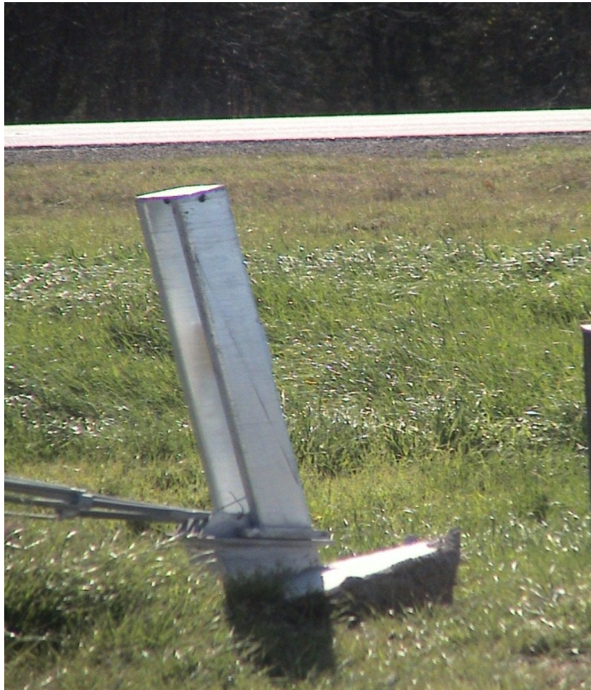
Figure A.2 Foundation Failures of 3-cable Median Barriers Built on Expansive Soils at IH 20 Westbound Sta. 1196+92
