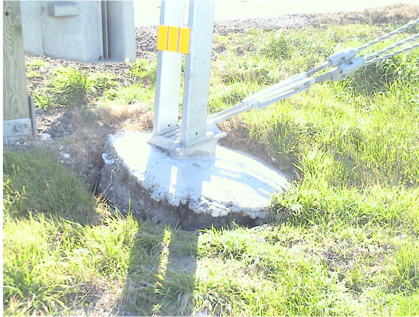
Figure 2.5 Foundation Failures of 3-cable Median Barriers Built on Expansive Soils at US 80 Eastbound Sta. 77+37
