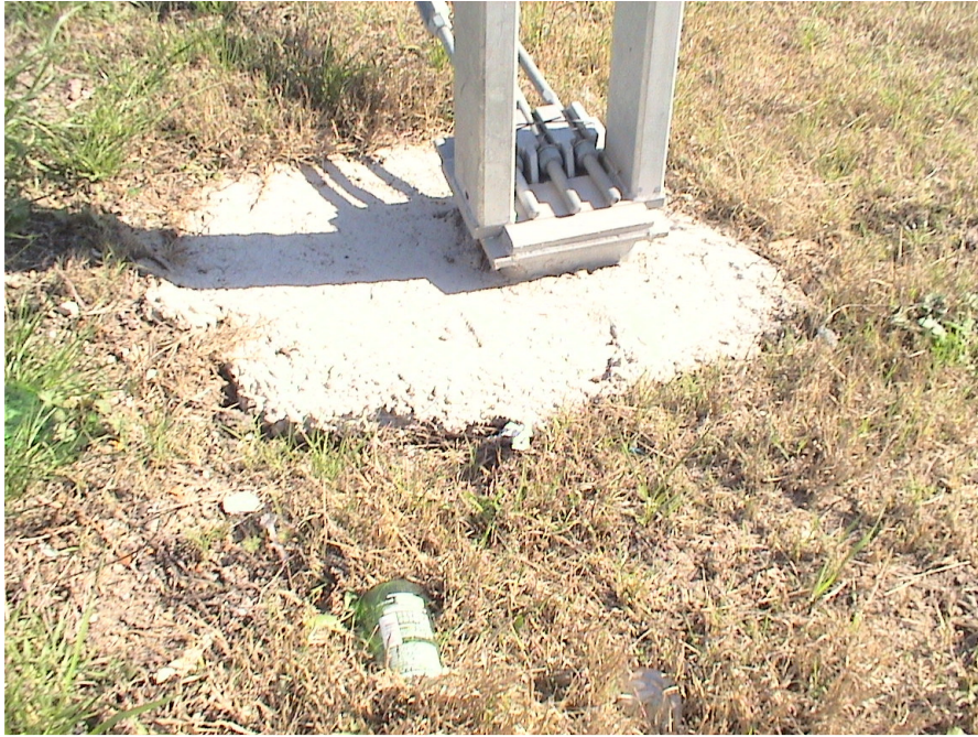
Figure A.28 Foundation Failures of 3-cable Median Barriers Built on Expansive Soils at US 80 Westbound Sta. 114+24
