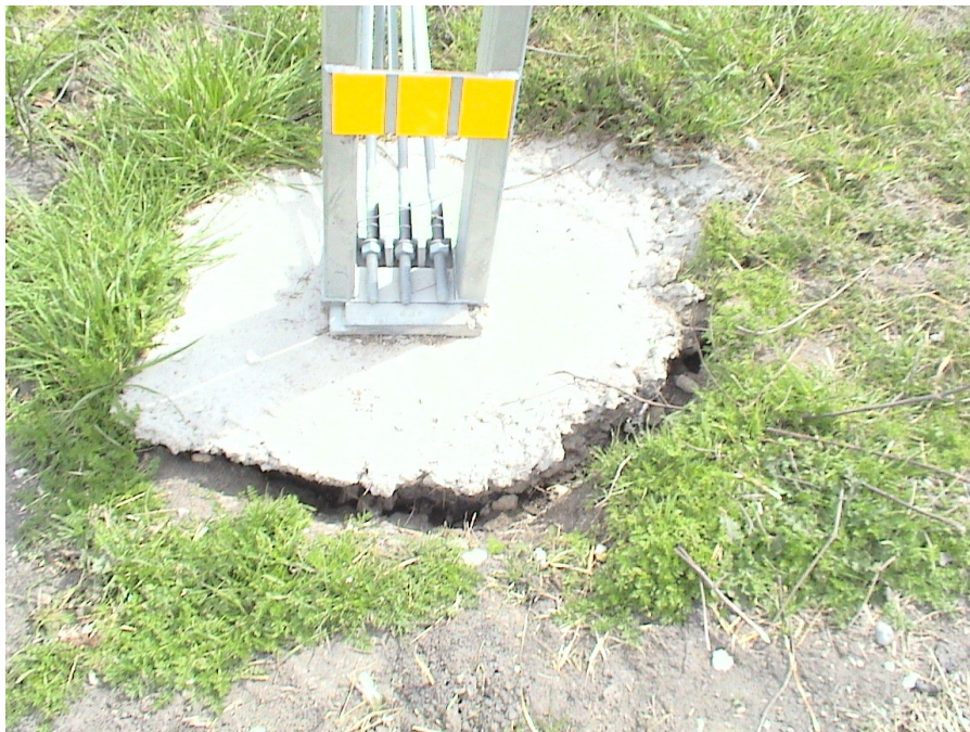
Figure A.35 Foundation Failures of 3-cable Median Barriers Built on Expansive Soils at US 80 Eastbound Sta. 486+78
