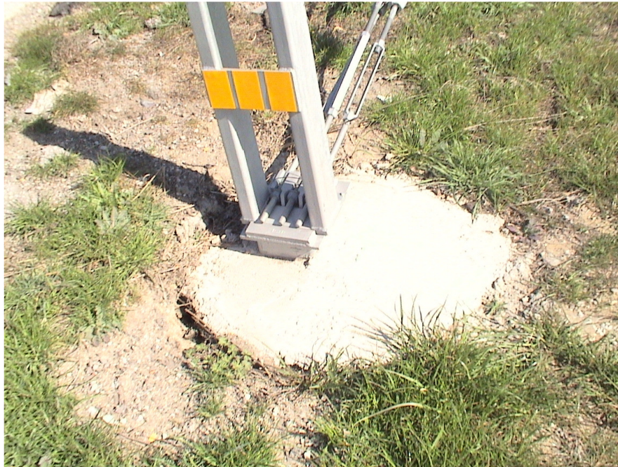
Figure A.30 Foundation Failures of 3-cable Median Barriers Built on Expansive Soils at US 80 Westbound Sta. 124+51
