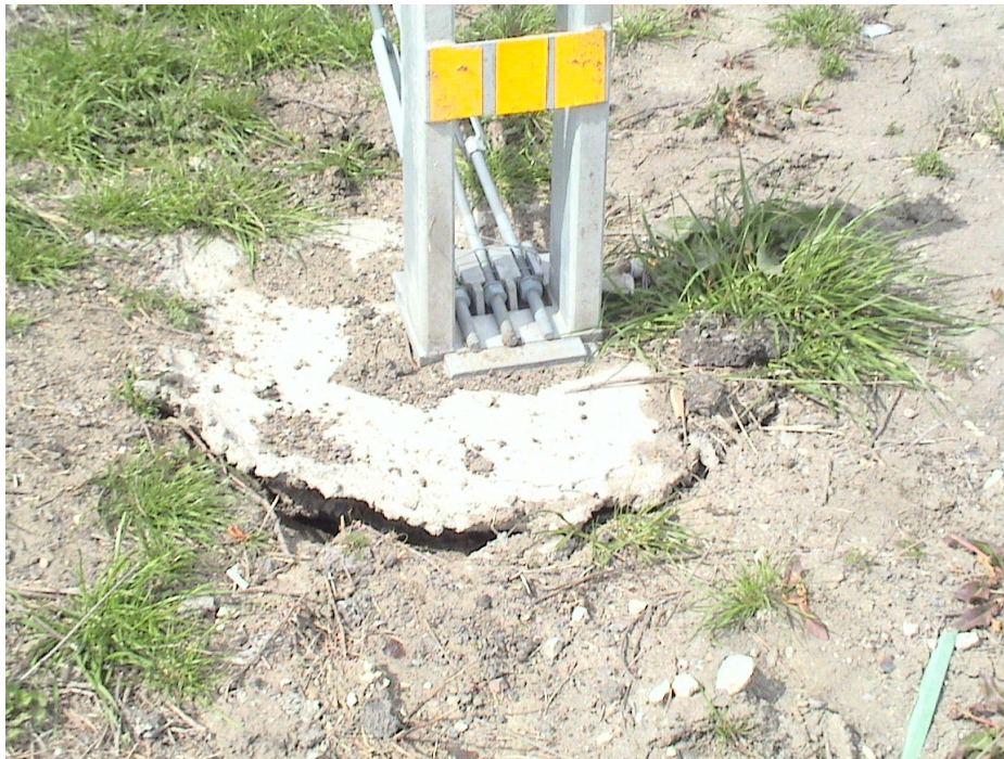
Figure A.36 Foundation Failures of 3-cable Median Barriers Built on Expansive Soils at US 80 Eastbound Sta. 493+07
