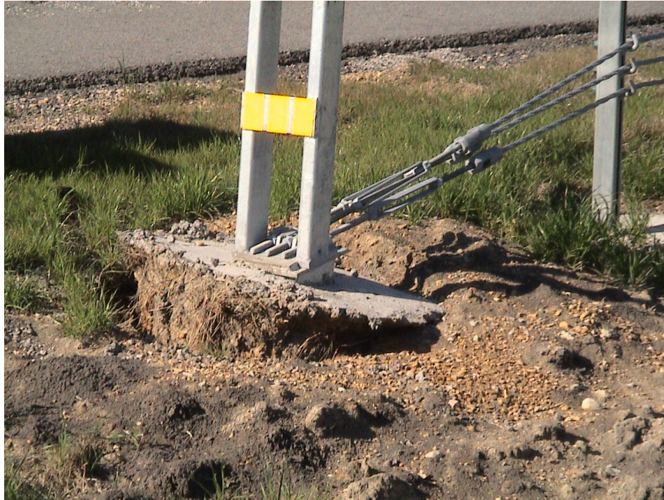
Figure 1.2 Typical Foundation Failures of 3-cable Median Barriers Built on Expansive Soils at US 175 Eastbound Sta. 149+98
