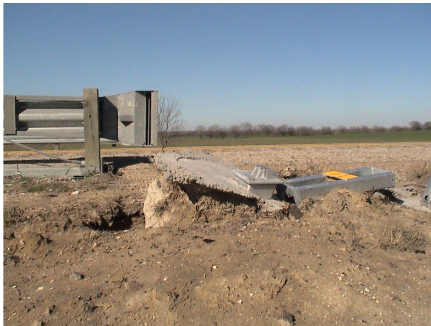
Figure A.8 Foundation Failures of 3-cable Median Barriers Built on Expansive Soils at IH 20 Westbound Sta. 993+50
