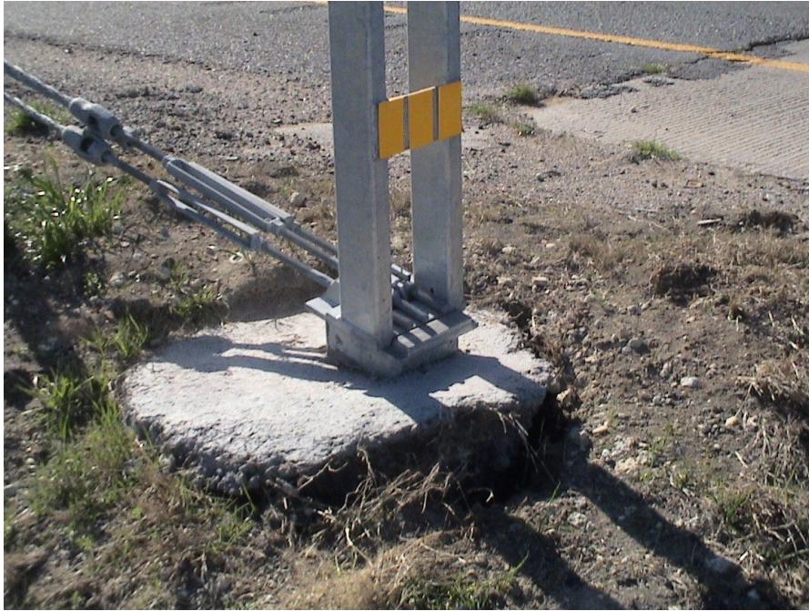
Figure A.11 Foundation Failures of 3-cable Median Barriers Built on Expansive Soils at US 175 Eastbound
