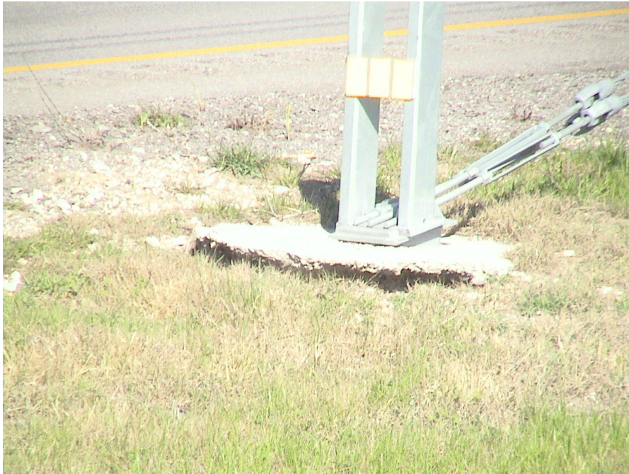
Figure A.24 Foundation Failures of 3-cable Median Barriers Built on Expansive Soils at US 80 Westbound Sta. 81+93
