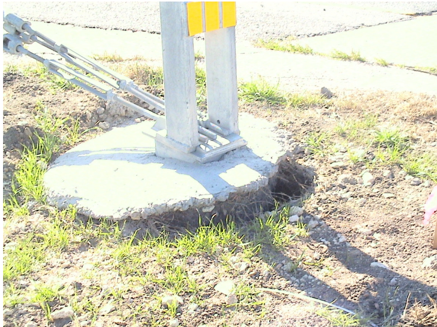
Figure 2.4 Foundation Failures of 3-cable Median Barriers Built on Expansive Soils at US 175 Eastbound Sta. 92+00
