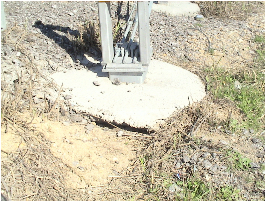
Figure A.17 Foundation Failures of 3-cable Median Barriers Built on Expansive Soils at US 80 Westbound Sta. 37+58
