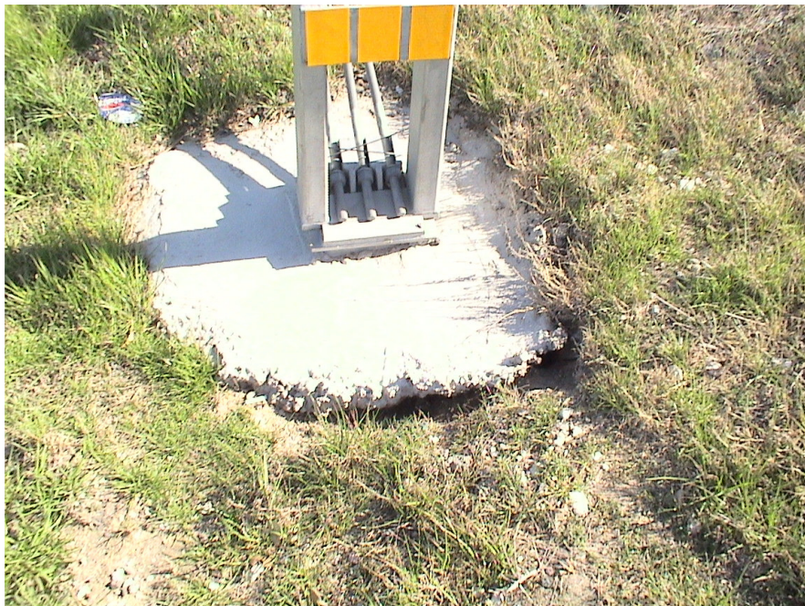
Figure A.27 Foundation Failures of 3-cable Median Barriers Built on Expansive Soils at US 80 Eastbound Sta. 113+79
