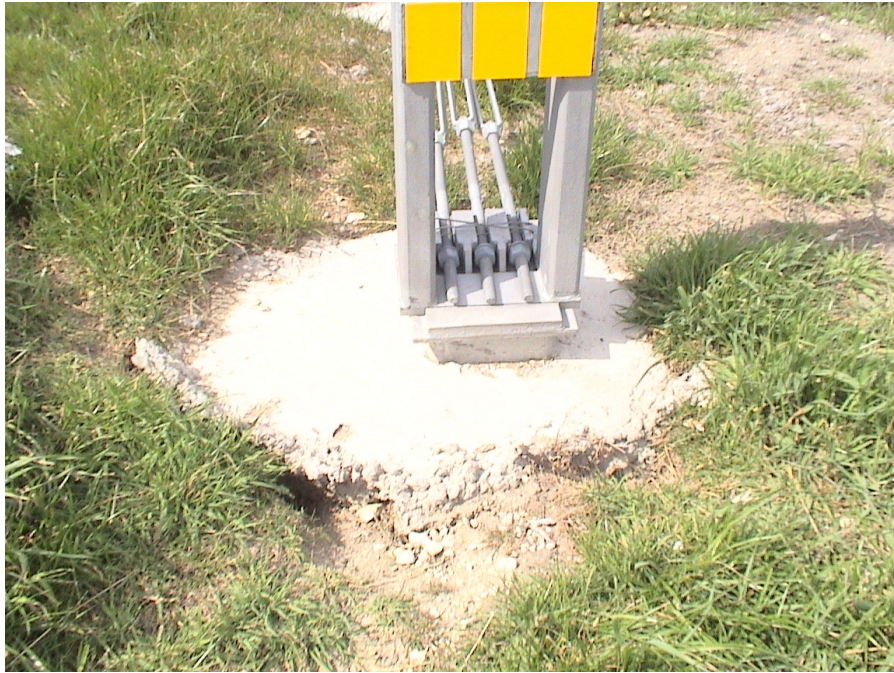
Figure A.32 Foundation Failures of 3-cable Median Barriers Built on Expansive Soils at US 80 Eastbound Sta. 462+95
