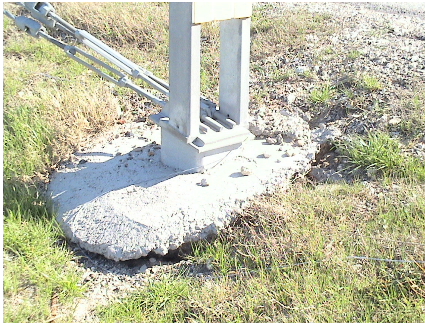
Figure A.19 Foundation Failures of 3-cable Median Barriers Built on Expansive Soils at US 80 Eastbound Sta. 64+28
