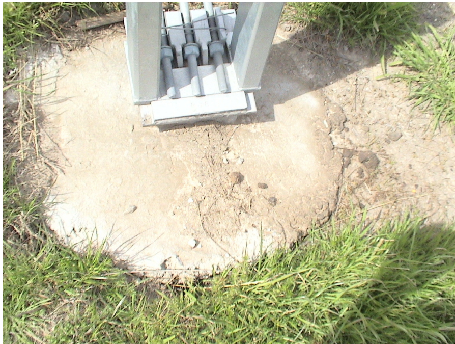
Figure A.34 Foundation Failures of 3-cable Median Barriers Built on Expansive Soils at US 80 Eastbound Sta. 483+70
