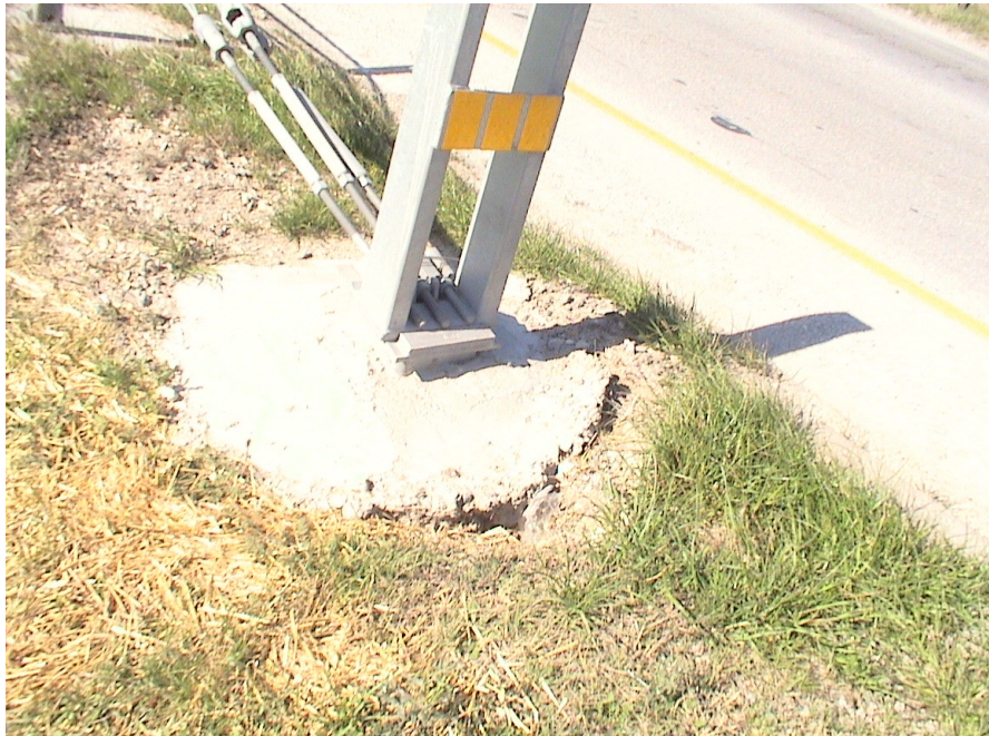
Figure A.29 Foundation Failures of 3-cable Median Barriers Built on Expansive Soils at US 80 Westbound Sta. 120+90
