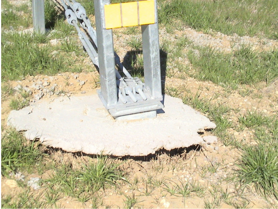
Figure A.15 Foundation Failures of 3-cable Median Barriers Built on Expansive Soils at US 175 Eastbound Sta. 658+15
