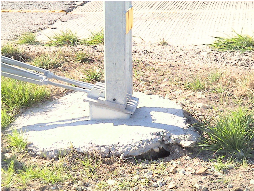
Figure A.13 Foundation Failures of 3-cable Median Barriers Built on Expansive Soils at US 175 Eastbound Sta. 137+62
