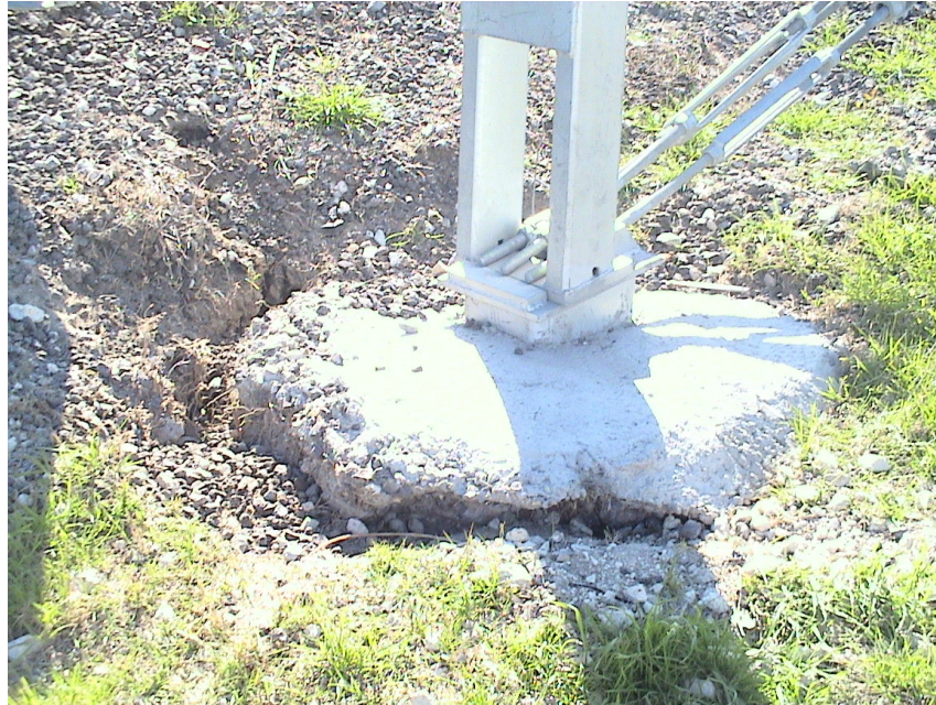
Figure A.18 Foundation Failures of 3-cable Median Barriers Built on Expansive Soils at US 80 Eastbound Sta. 46+68
