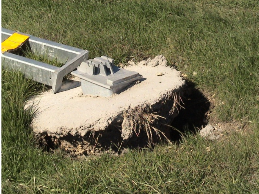
Figure A.4 Foundation Failures of 3-cable Median Barriers Built on Expansive Soils at IH 20 Westbound Sta. 1069+00
