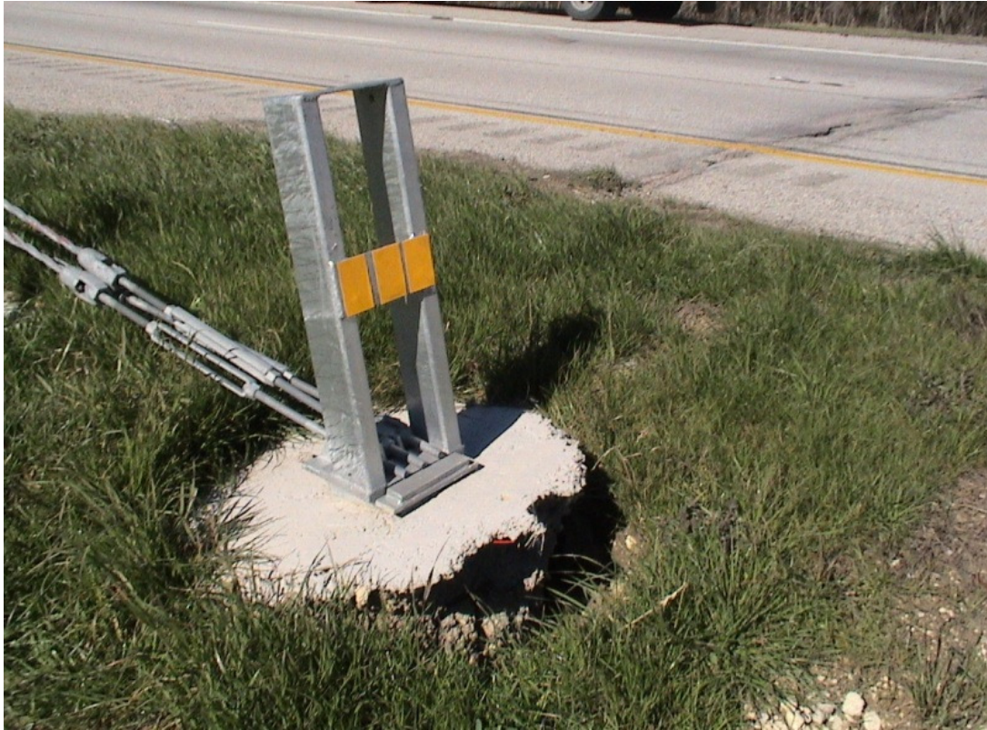
Figure 1.1 Typical Foundation Failures of 3-cable Median Barriers Built on Expansive Soils at IH 20 Westbound Sta. 1338+57
