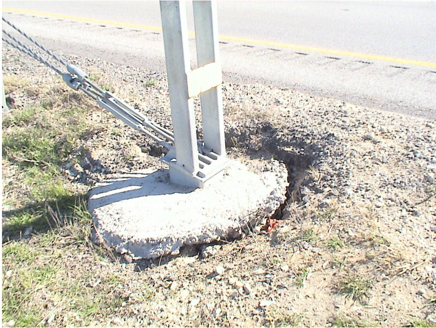
Figure A.16 Foundation Failures of 3-cable Median Barriers Built on Expansive Soils at US 80 Eastbound Sta. 37+29
