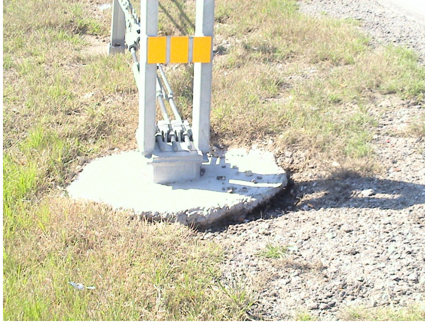
Figure A.22 Foundation Failures of 3-cable Median Barriers Built on Expansive Soils at US 80 Westbound Sta. 77+07
