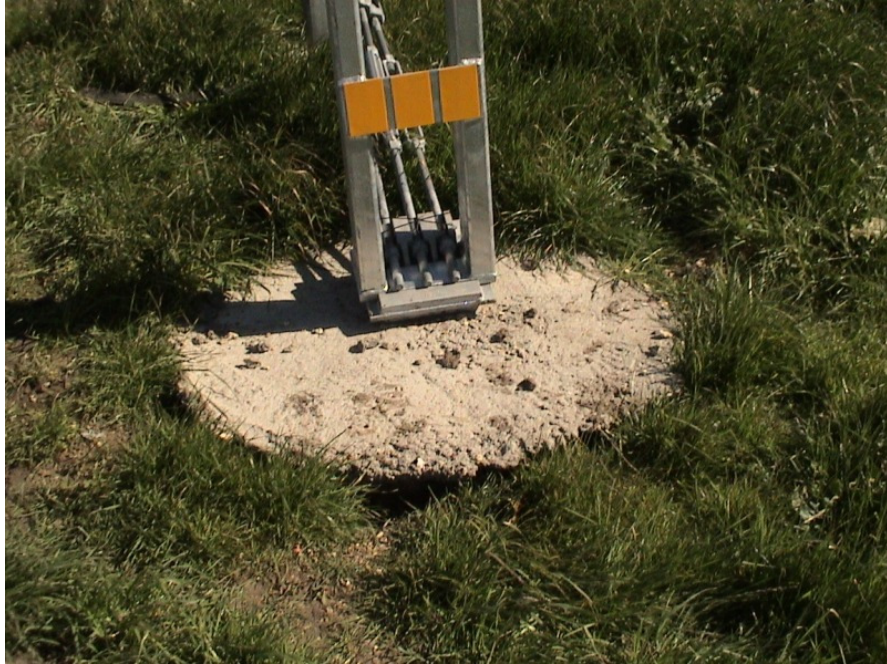
Figure A.3 Foundation Failures of 3-cable Median Barriers Built on Expansive Soils at IH 20 Westbound Sta. 1071+00
