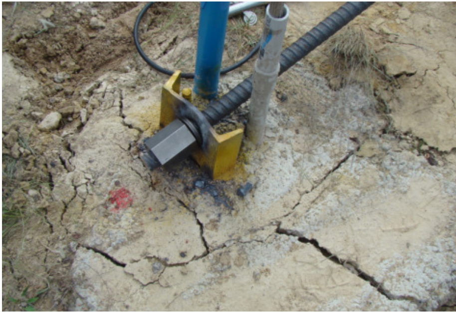
Figure 5.2 Cracking in Concrete Material
