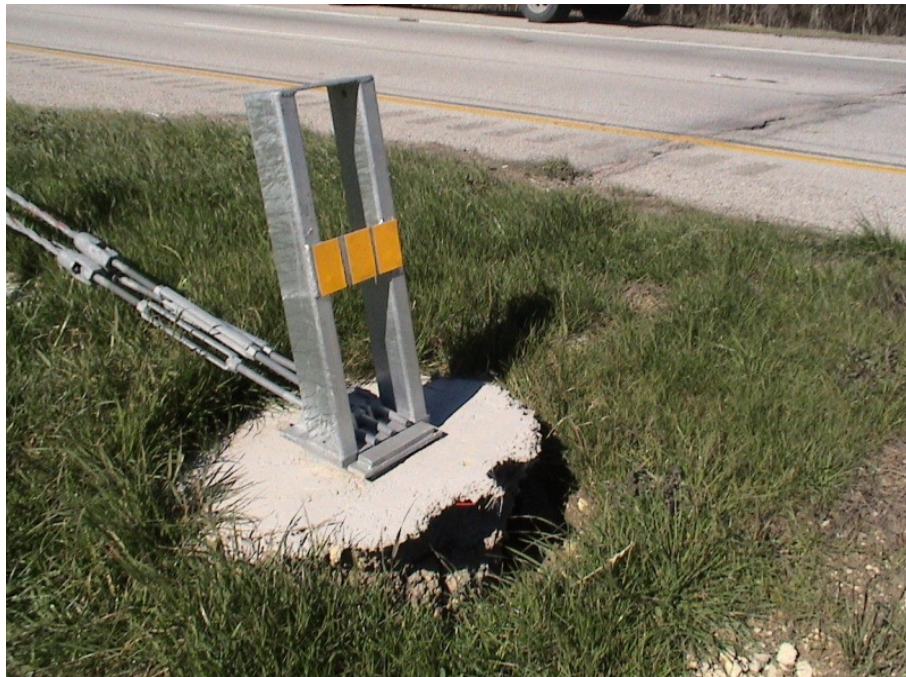
Figure A.1 Foundation Failures of 3-cable Median Barriers Built on Expansive Soils at IH 20 Westbound Sta. 1338+57
