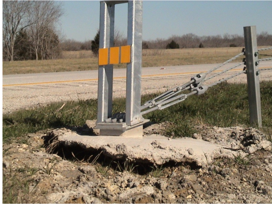
Figure A.7 Foundation Failures of 3-cable Median Barriers Built on Expansive Soils at IH 20 Westbound Sta. 846+92
