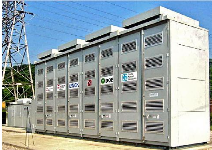
Figure 3.6 1MW NAS Battery Installation in Charleston, W.V. [37]
