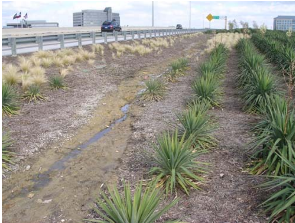
Figure 22. Weeping Love Grass and Soft-tip Yucca struggling in the drainage swale (Scott, Fall/2006.)
