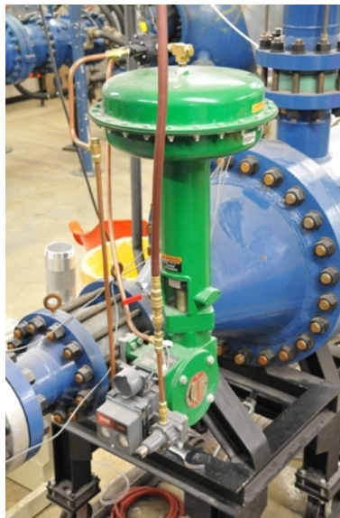
Figure 3.4. SSWT control valve.
