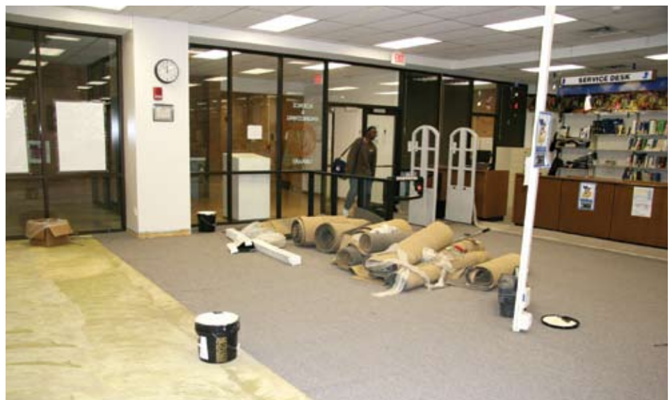
The Science and Engineering Library received the gift of more space when 80,000 volumes were relocated to the LCD. New carpet was installed before furniture was put in place for staff and an additional study group area.
