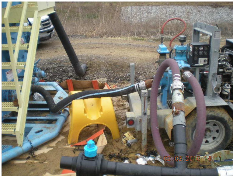
Figure 3.5: Leachate storage tank and pumping station (City of Denton, MSW landfill)
