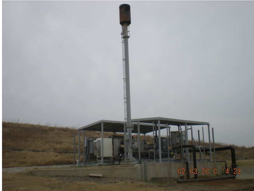
Figure 3.16: Landfill gas flare station, MSW Landfill, City of Denton
