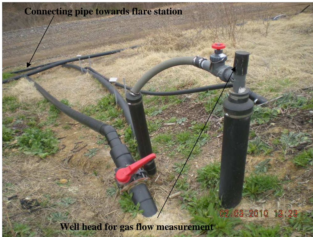
Figure 3.17: Gas well head and connection pipe towards well head
