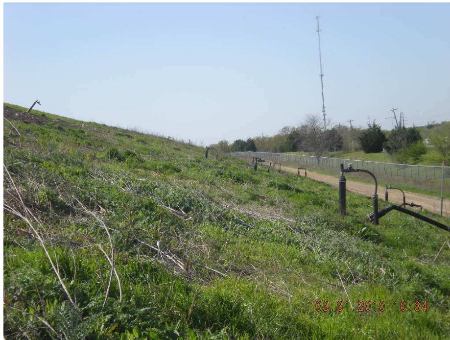
Figure 3.12: Interconnected leachate recirculation pipes in landfill
