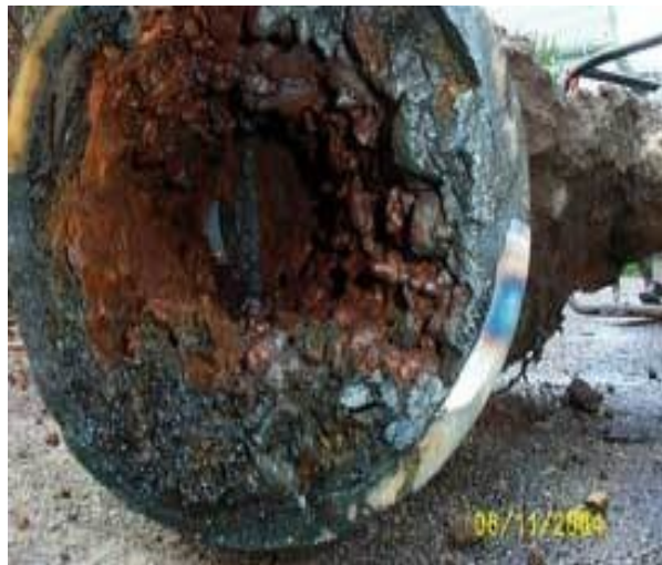
Figure 1.7 - Intensity of Tuberculation Present (Source: 3M Water Infrastructure)
