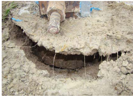
Figure 6.14. Test Shaft Concrete Broken Horizontally
