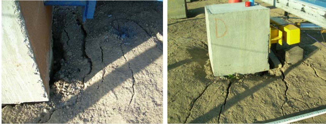
Figure 2.33. Typical Cracks After Testing (Pierson et al., 2009)
