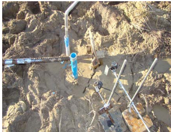
Figure E.11. Winter Condition Test Shaft Concrete Failures
