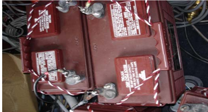
Figure 3.10 12- Volt deep cycle batteries
