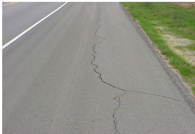
Figure 1.2 Longitudinal and Transverse Cracks Resulting from Pavement Distress at IH 820 N, Fort Worth, Texas
