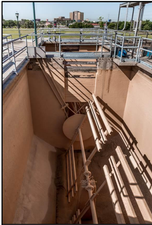
Figure 1.2: Typical Plant Flocculator (Stage 2)
