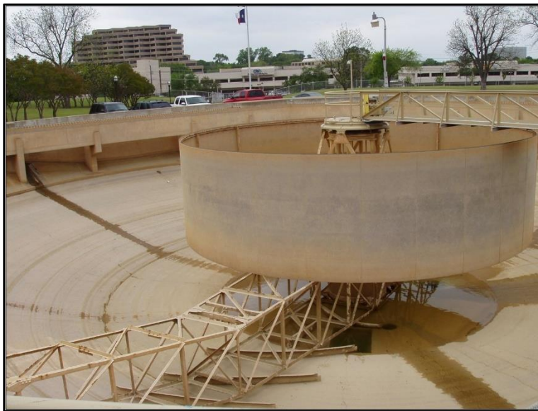
Figure 1.3: Typical Plant Clarifier
