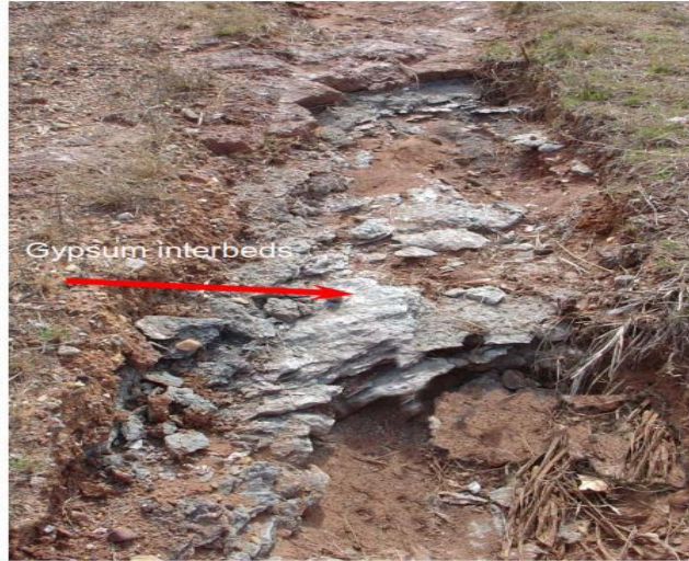
Figure 2-2: East side of the project area has a heaved area. (Chen et al. 2005)
