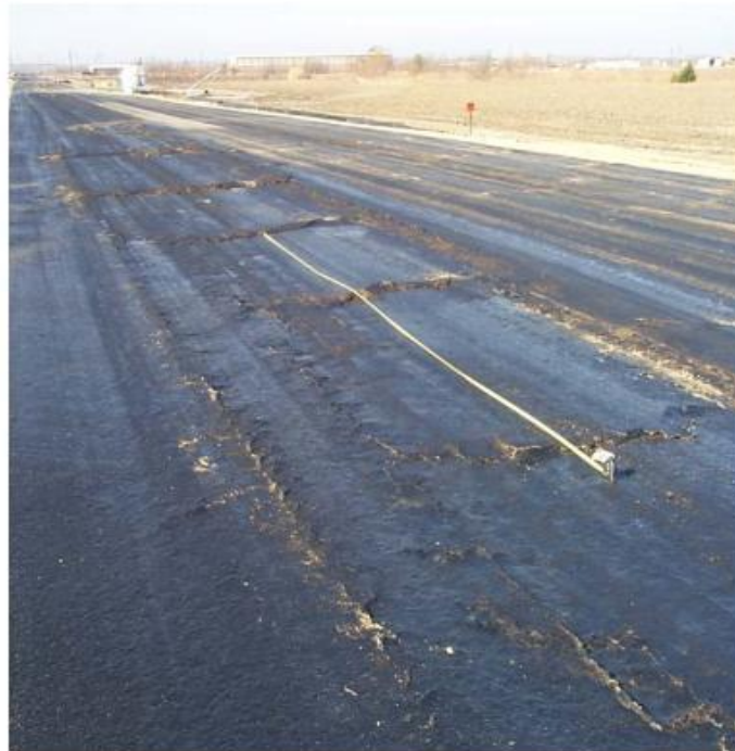
Figure 2-4: Near Midlothian, Texas, a Heave on US 67 (Wimsatt 1999)
