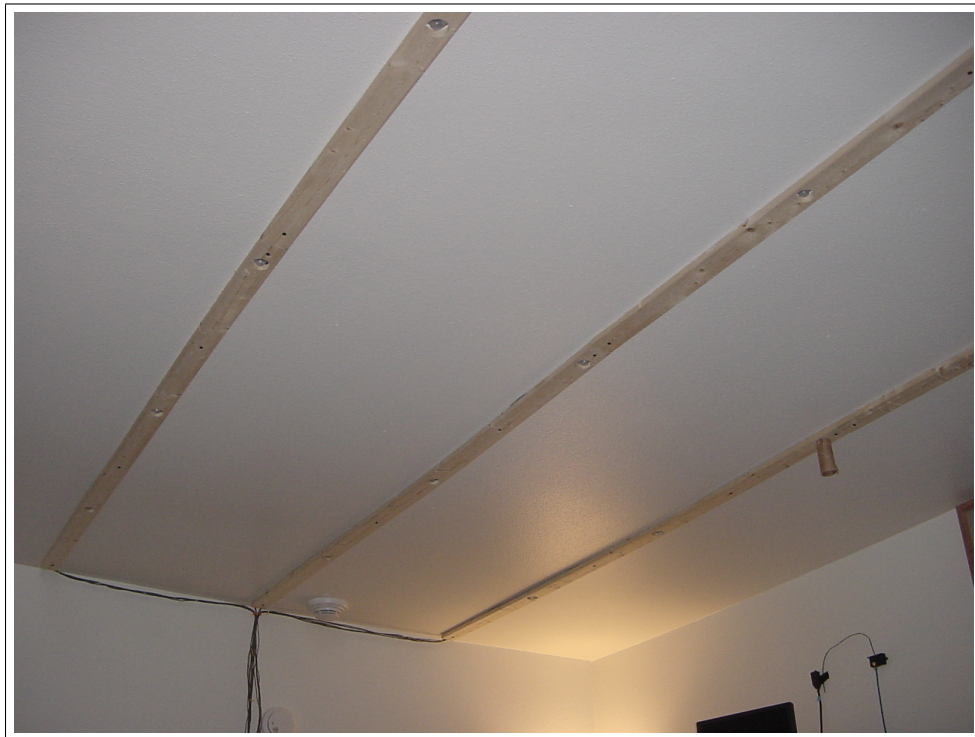
Figure C.7. ArgusD ceiling mounted PIR motion sensors.
