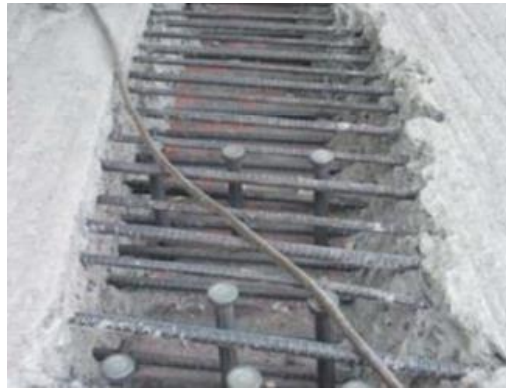
Figure 2- 23: Headed studs welded to the steel girder after water blasting (Collin, et al., 2015)
