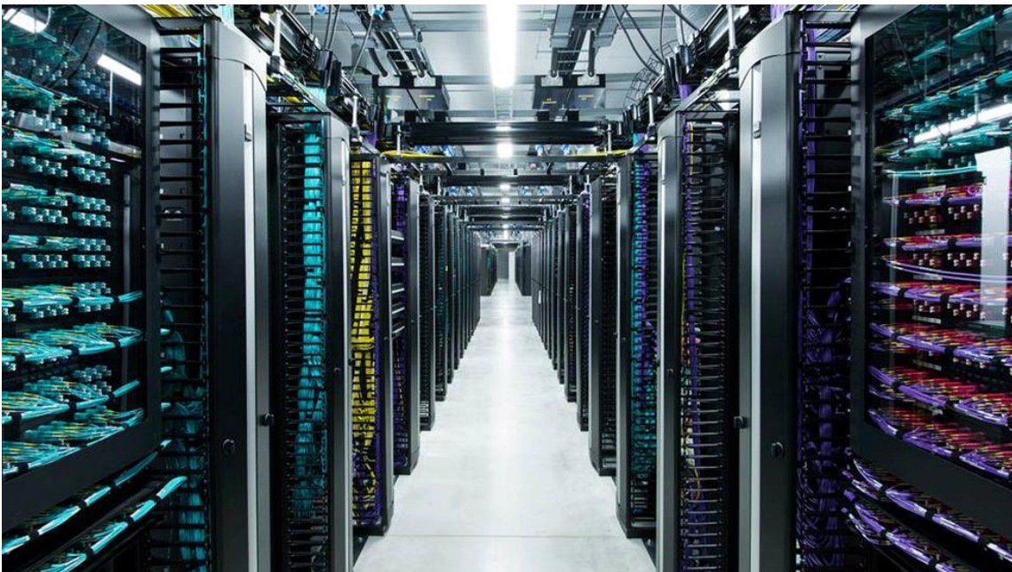
Figure. 1.1 Facebook Datacenter room
