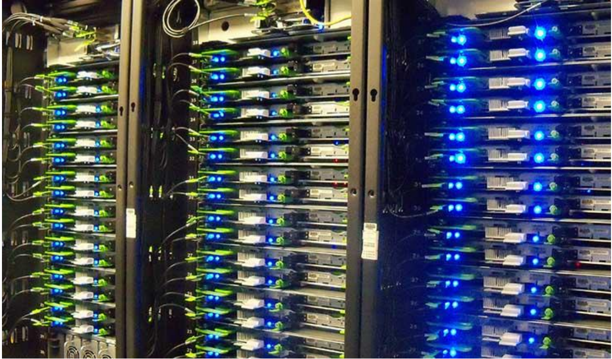
Figure 1 High Density Facebook Data Center
