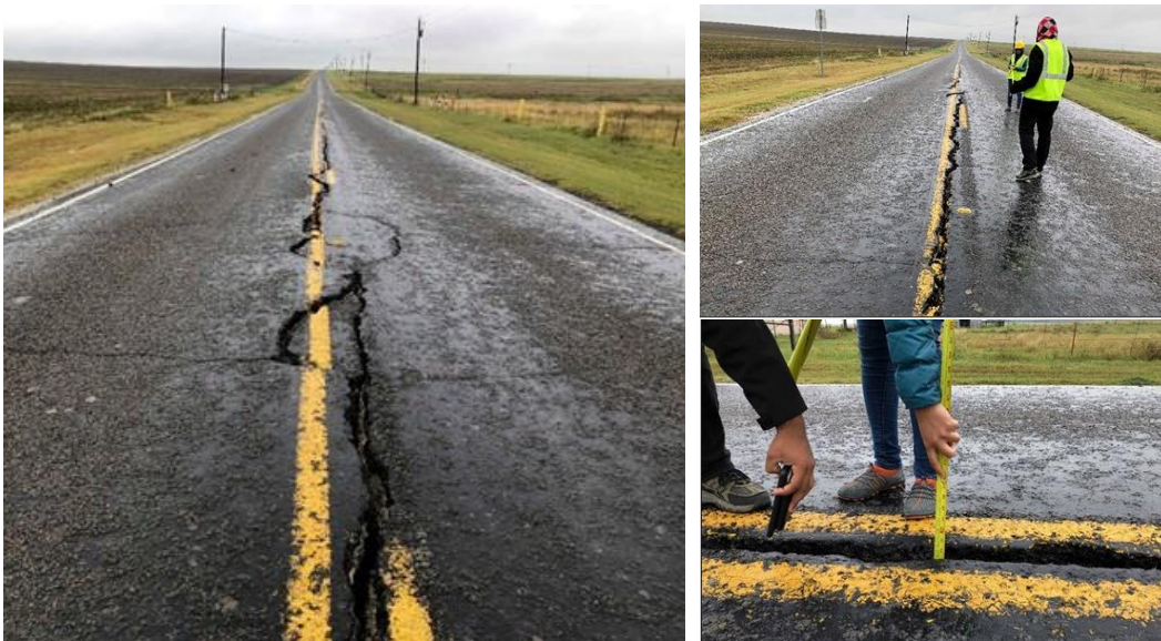
Figure 3–2 Observed Pavement Distresses During Initial Field Inspection
