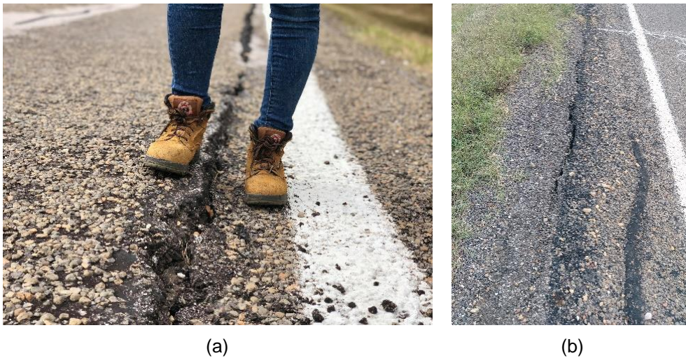
Figure 2-5 (a) Edge Drop and (b) Longitudinal Cracks due to Expansive Subgrade Soil
