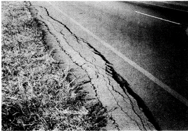
Figure 2–37 Crack at Pavement Edge after Installing Vertical Barrier (Steinberg, 1989)
