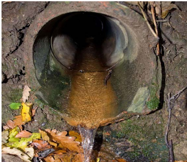
Figure 1-1 A Sample of Aging Underground Pipeline Source: Melissa Thompson Available at: https://newsblaze.com
