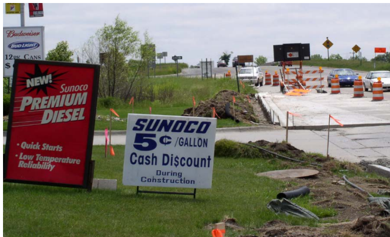
Figure 3-10 Business Loss due to Open-cut Pipeline Replacement Source: Najafi and Gokhale, 2005
