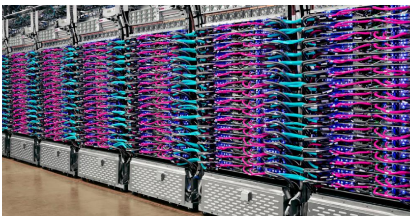
Figure 1. 4 google liquid cooled rack for Machine learning[6]
