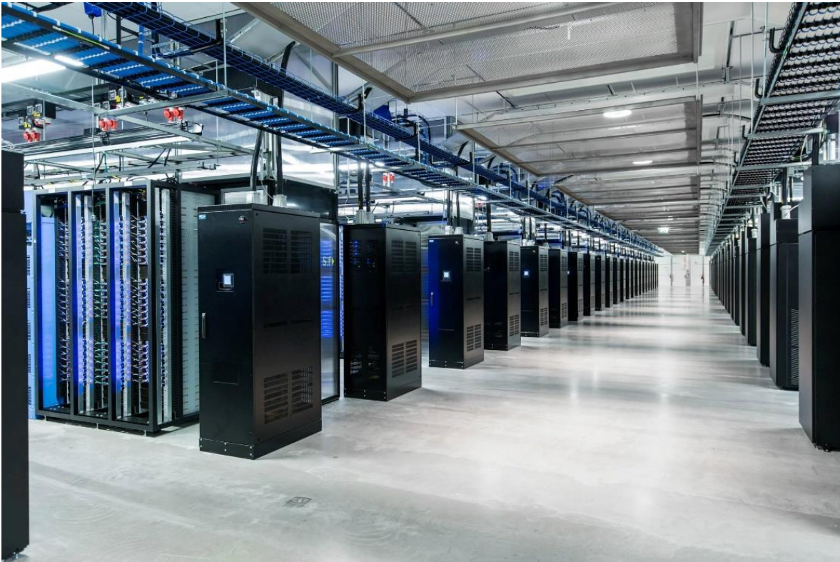
Figure 1. 1 Facebook's Data Center at Lulea, Sweden[3]
