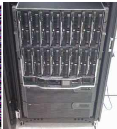
Figure 1. 5 HP C7000 rack[7]
