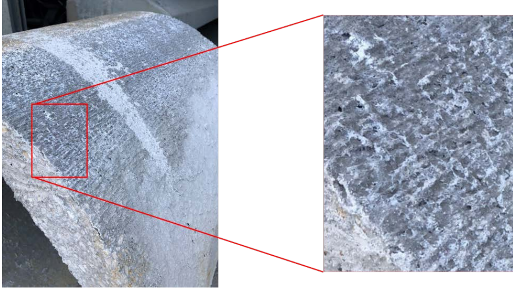
Figure 76. Gypsum formation on the immersed pipe surface, pH2-T50 for five months
