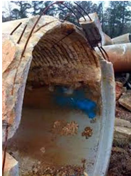
Figure 8. Steel corrosion in an RCP
