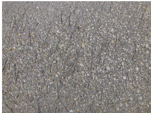
Figure 86. Exposed synthetic fibers in the pH2-T50 pipe after one year
