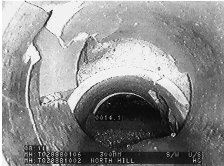
Figure 9. CCTV image of collapsed sewer pipes [3]
