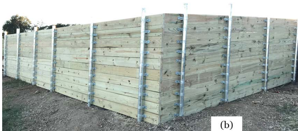
Figure 3. 56 (a) Sawing to shape and connecting corners using screws; (b) Complete wall facing of the test section.
