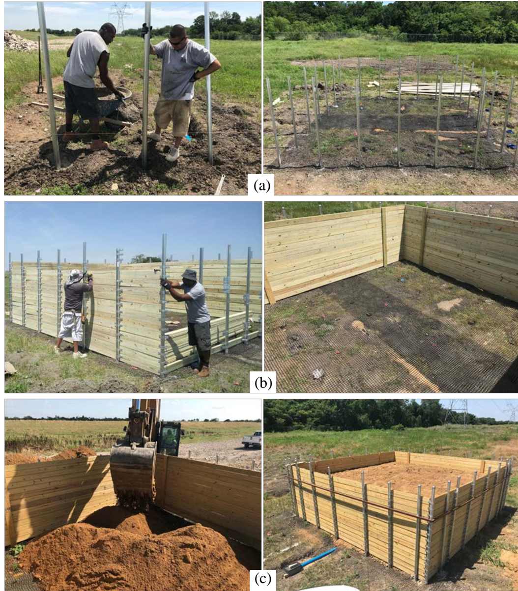
Figure 3. 53 Phase – II construction: (a) Installation of steel post and geogrid placement; (b) Connecting wooden planks with the post and wall construction; (c) Loading the test sections and completed test section.
