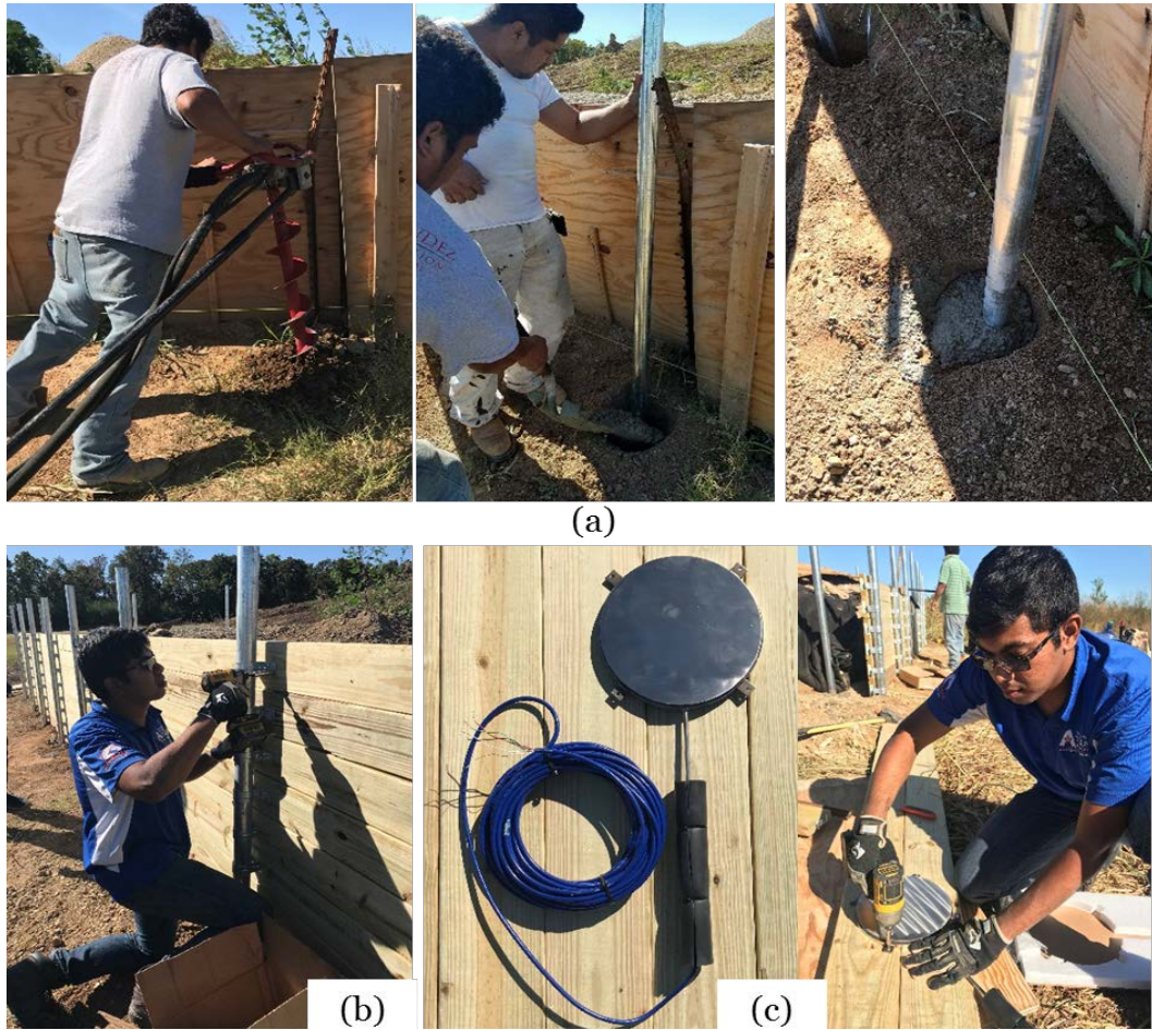
Figure 3. 55 (a) Installation of steel post; (b) Connecting wooden planks with the post; (c) Installing pressure sensor at the inside face of the wall facing.
