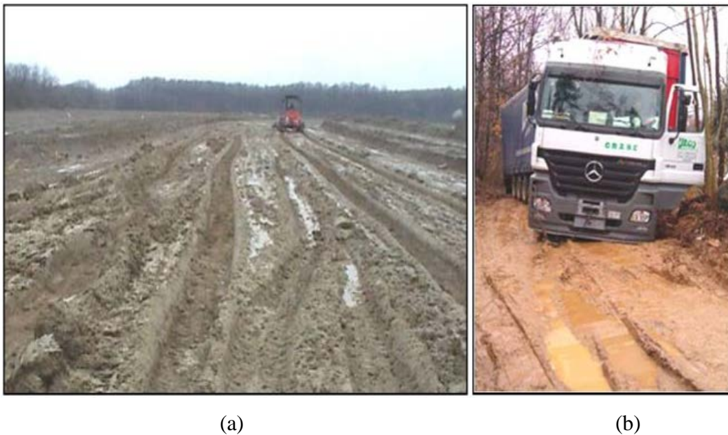
Figure 2. 1 (a) Construction work on soft soil; (b) Truck sinking into a soft soil road.
