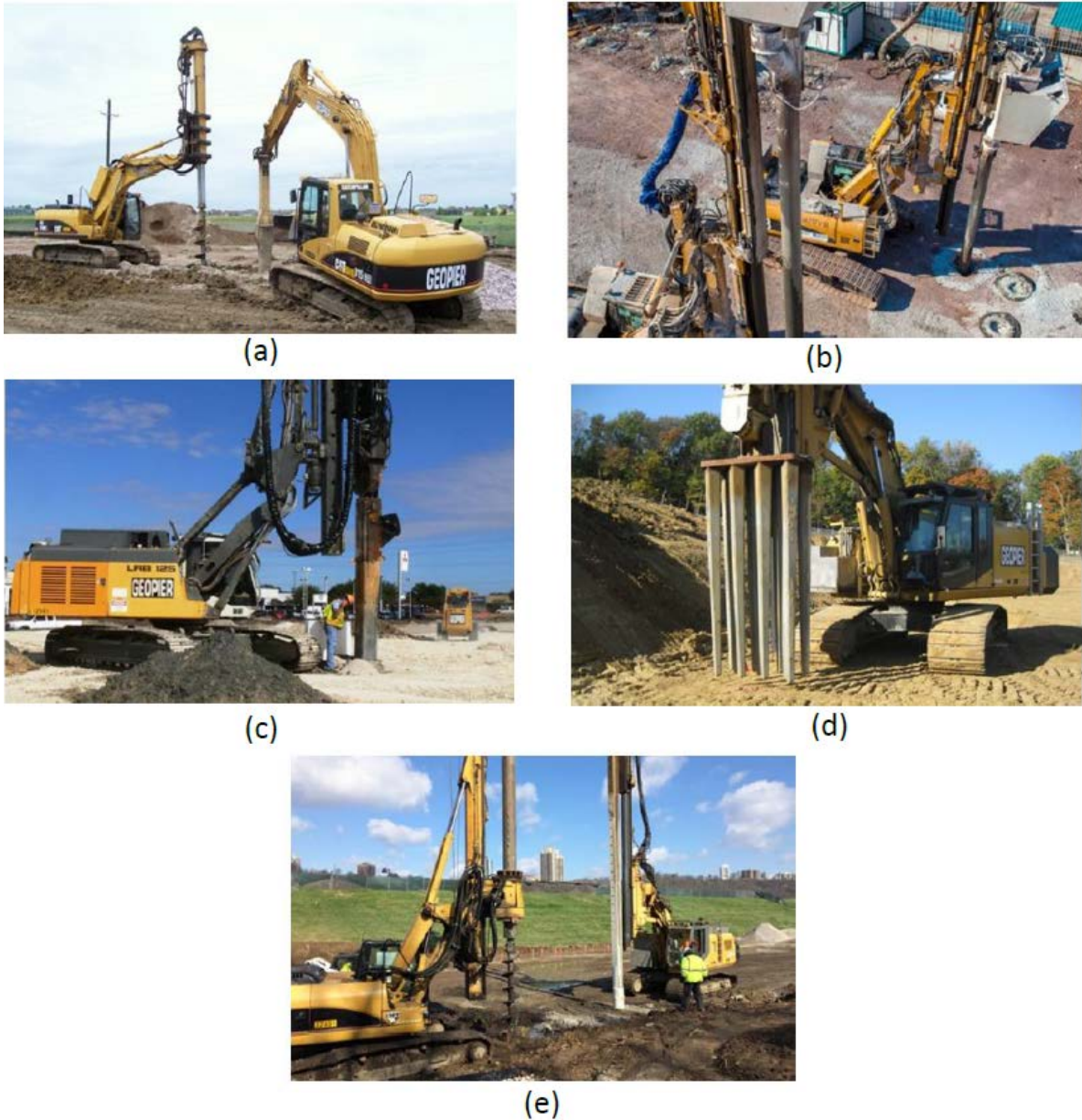
Figure 2. 11 Rammed Aggregate Pier Systems. (a) GP3 system; (b) Impact system; (c) Rampact system; (d) Densipact system; (e) X1 system ( www.Geopier.com ).
