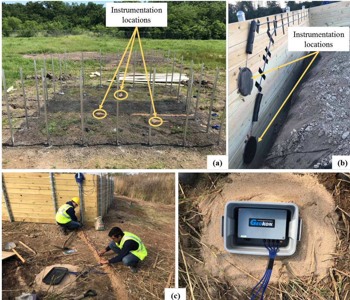
Figure 3.52 Data collection: Instrumentation locations for (a) vertical loaded test section, (b) lateral loaded test section; (c) data logger setup.
