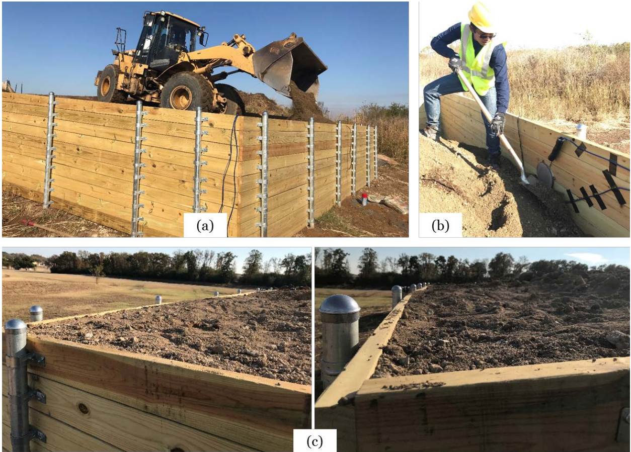
Figure 3. 57 (a) Backfilling test section; (b) Manually spreading soil near the facing; (c) Complete wall after backfilling.
