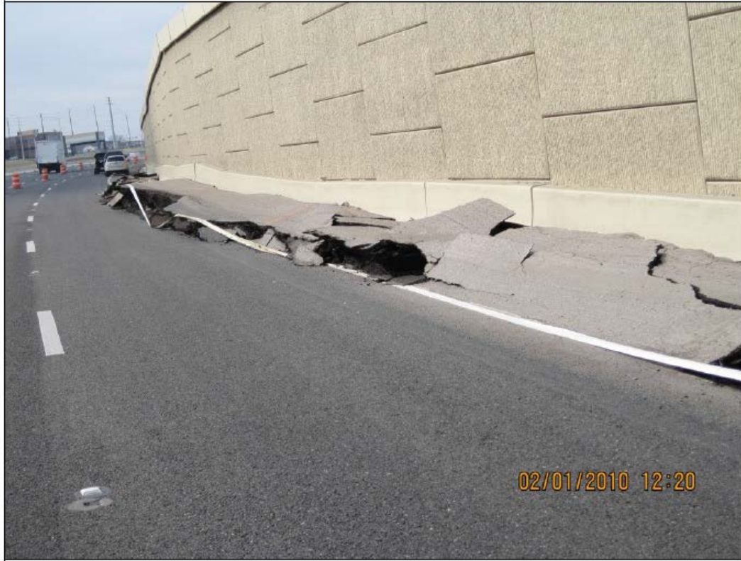
Figure 2. 55 Distress in pavement structure resulting from the lateral movement of MSE wall base (Schmidt and Harpstead, 2011).
