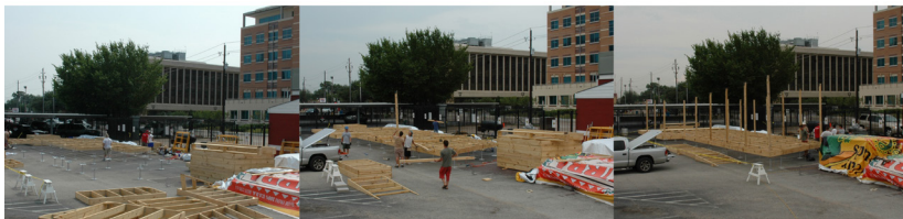
Southside on Lamar Pavilion under construction in Dallas. Photographs courtesy of Heath MacDonald.
