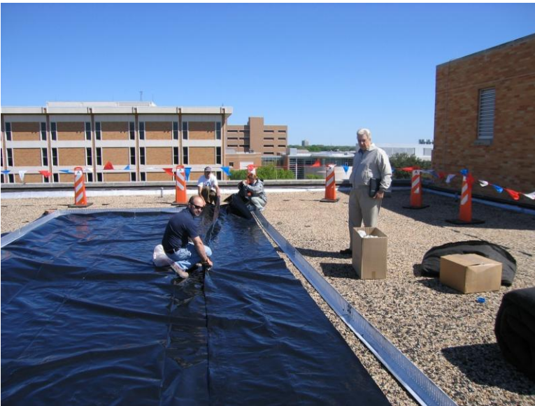
Figure 5: Installation of root barriers as Robert Nickel, of American Hydrotech, looks on
