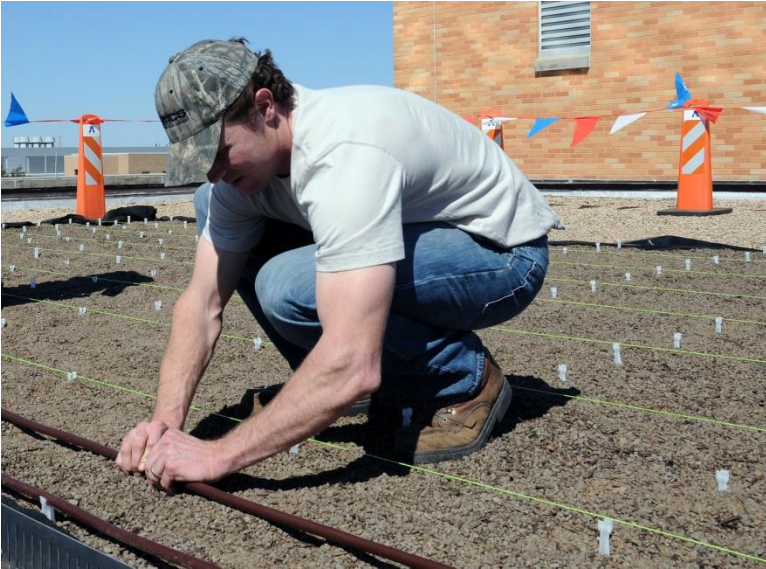
Figure 9: Netafim Drip Irrigation lines are snapped into 3-1/2 inch plastic rebar risers
