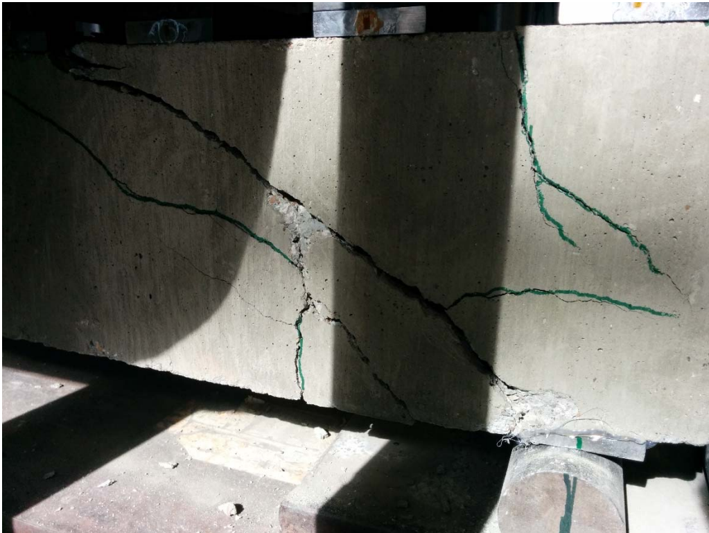
P5. Shear Cracking (continued)
