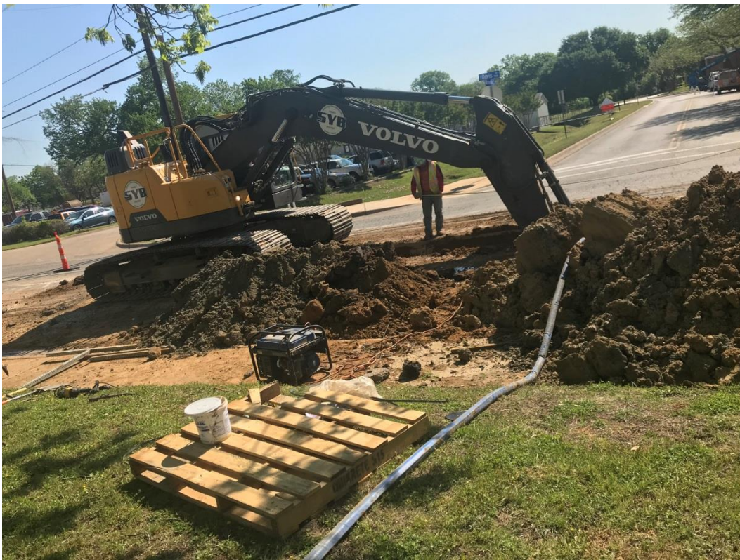
Fig. E3. Trenches dug to the curb after pavement is cut to trench width using a pavement saw
