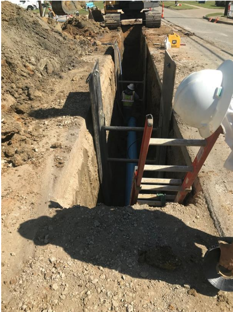
Fig. E5. Installation of pipe after trenching and supporting the lateral soil
