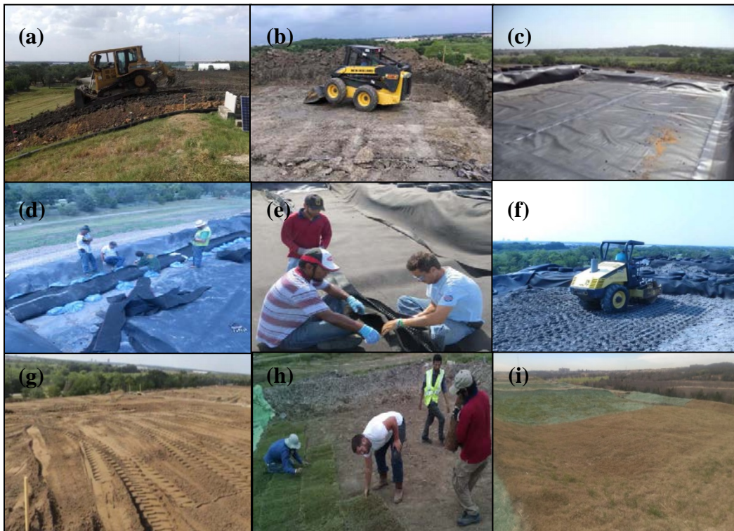
Figure 3-2 Steps of Lysimeter Construction (a) Embankment construction, (b) Embankment excavation, (c) Geomembrane placement (d) Percolation collection system installation, (e) Geo-composite drain placement, (f) Compacted clay placement, (g) Topsoil placement, (h) Vegetation and erosion mat placement, (i) ET cover lysimeter after completion
