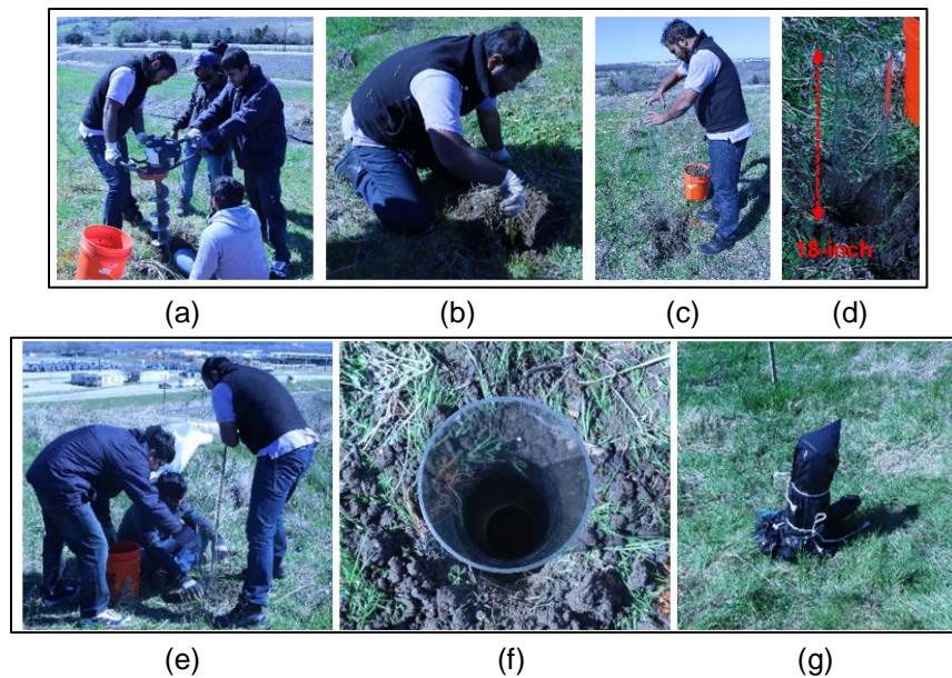
Figure 3.18 (a) Boring with spiral augur (b) measuring depth of hole (c) inserting plexiglass (d) top 18-inch of plexiglass (e) gap filling with soil between hole and outer wall of plexiglass and compaction (f) in-place plexiglass (g) temporary wrappedup plexiglass
