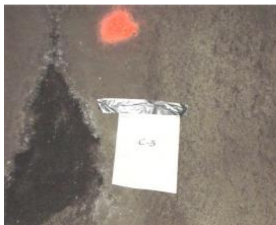
Figure Error! No text of specified style in document. -3 Distress region on tunnel lining (C-3), (Puppala et al.2010)
