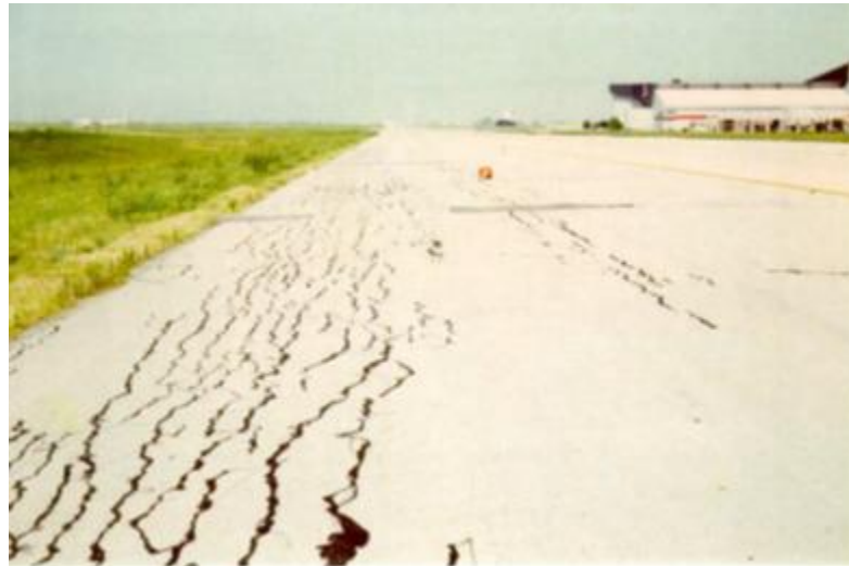
Figure Error! No text of specified style in document. -2 heave distress pattern on west shoulder of taxiway - (Reproduced from Talluri, 2013)
