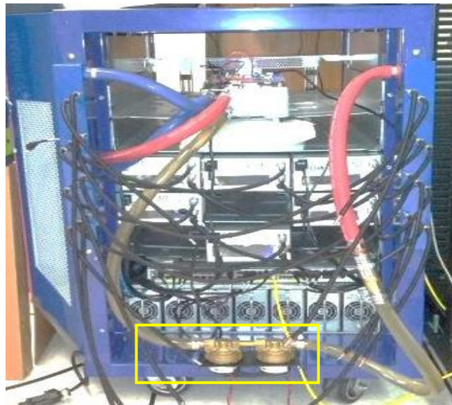
Figure 4-10: a) CHX 40 (left) replaced on the top of the rack with centralized pumps driving the flow in the system b) previous design of centralized system (right) - the location of the pumps are highlighted
