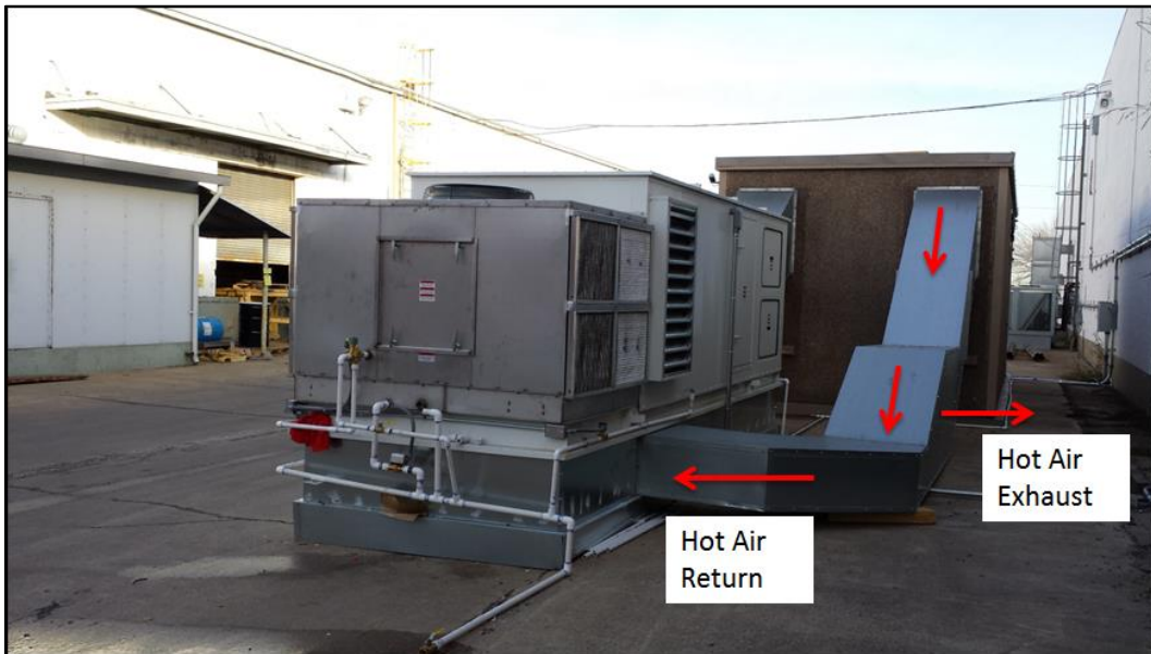
Figure 2-6 Modular Data Center: Shows Hot Data Center Return Duct
