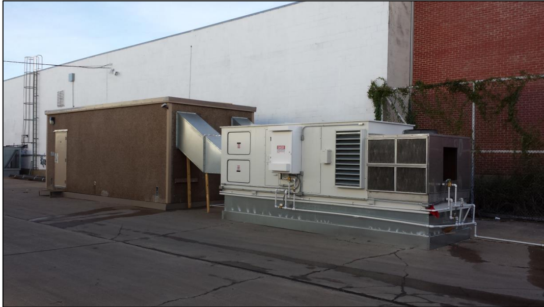
Figure 3-11 Test Bed Modular Data Center
