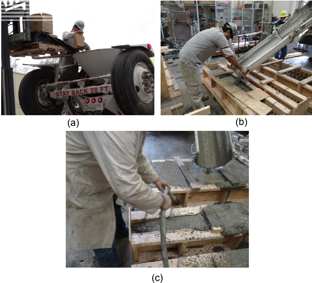
Figure 3.16 (a) dumping of steel fibers into the truck mixing drum; (b) shooting of SFRC mixture into formworks; (c) SFRC compactness
