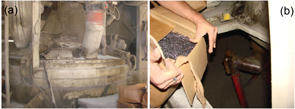
Figure 3.12 (a) a view of pan mixer in local Hanson Pipe & Precast Plant; (b) dumping of steel fibers into the mixer through the intended hatch
