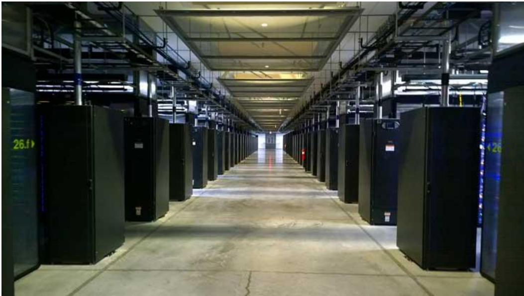
Figure 1-1 Facebook Data Center in North Carolina [1]
