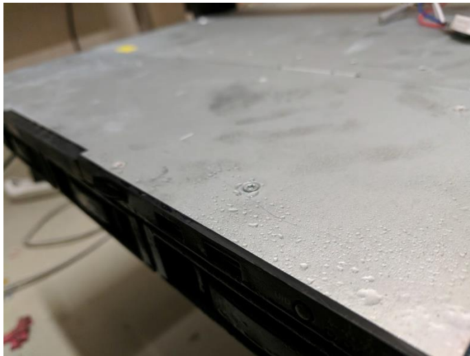
Figure 1 Condensation on IT equipment
