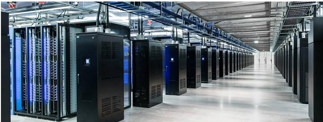
Figure 1-1 Facebook Data Center
