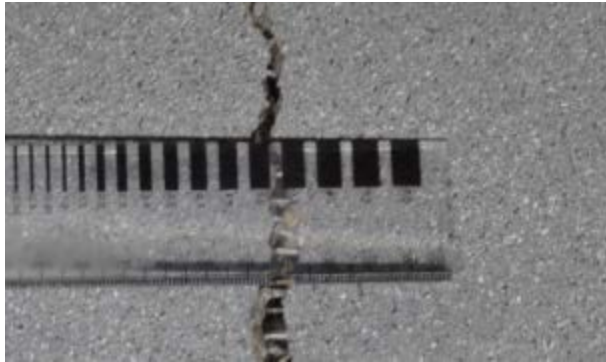
Figure 1-4 graduated scale (cracks' comparator)
