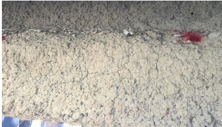
(a) Cracks on the surface of the insulation
