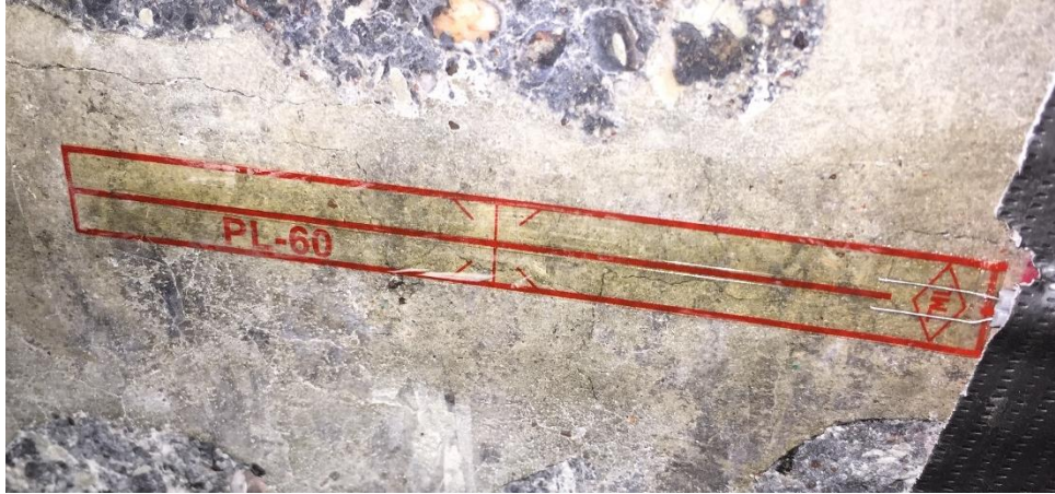
Figure 6-35 Cracks underneath the strain gauge
