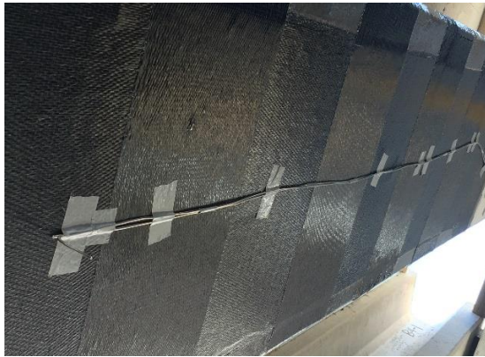
(m) Longitudinal FRP with Thermocouples installed at the Interface between the fire proofing and the FRP
