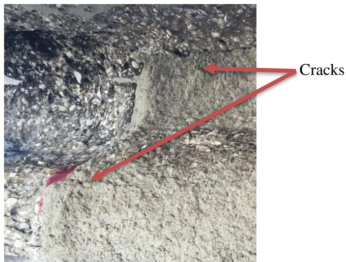
(b) Cracks emanating from termination point of fireproof
