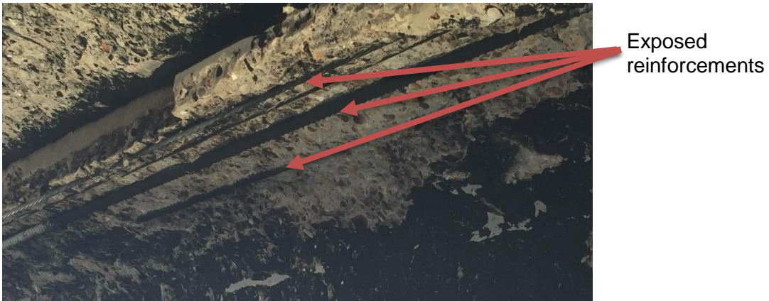
Figure 5-38 Exposed top reinforcements and strand for Girder-3
