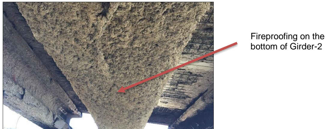
Figure 5-58 reference point used for measuring the elevation of the mid-span of Girder-2 after the fire
