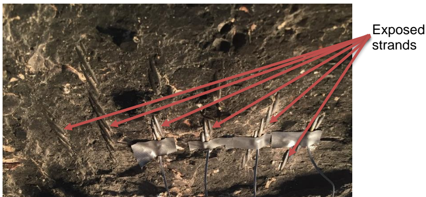
Figure 5-33 Exposed strands on Girder-2
