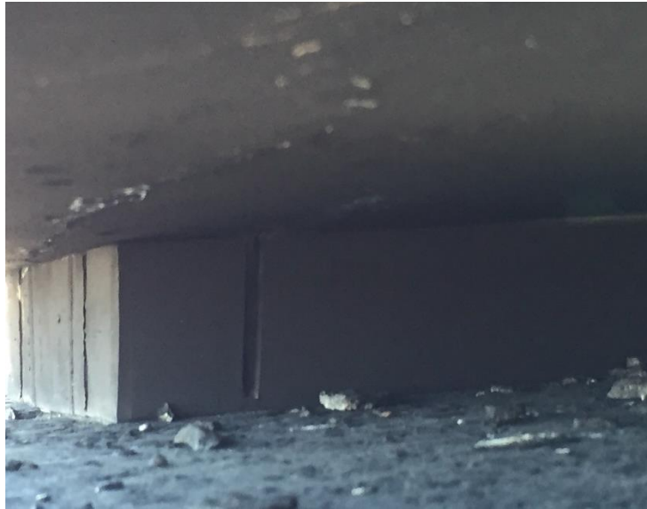
Figure 5-46 Deformation of bearing pad
