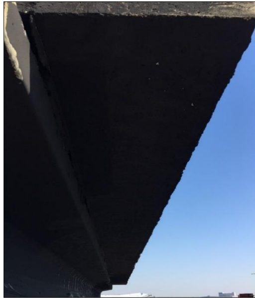
Figure 5-44 Overhang portion of the deck on Girder-3 side after the fire
