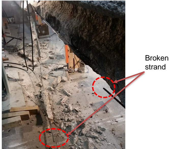
Figure 6-15 Broken prestressing strand
