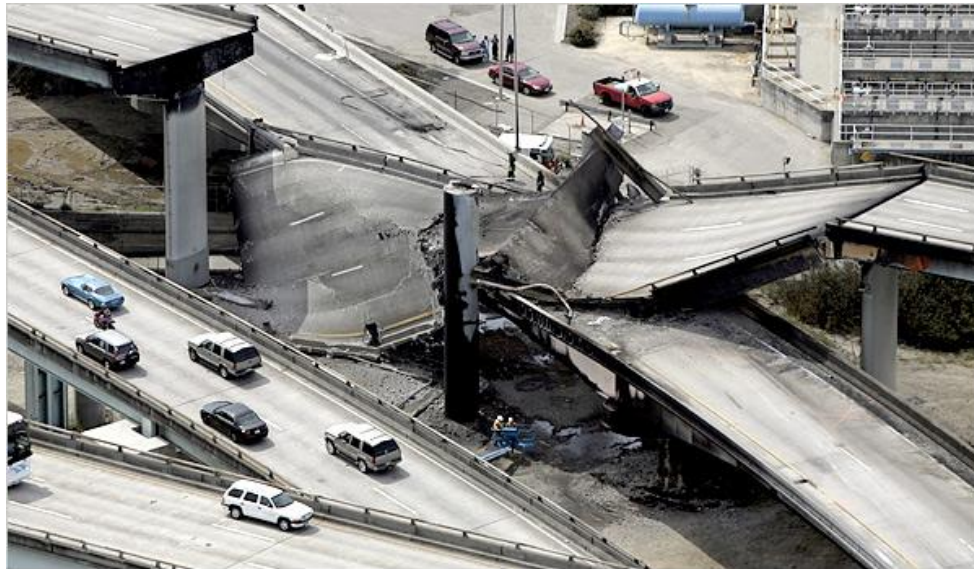
Figure 2-2 Collapsed MacArthur Maze Bridge (New York Times 2007)
