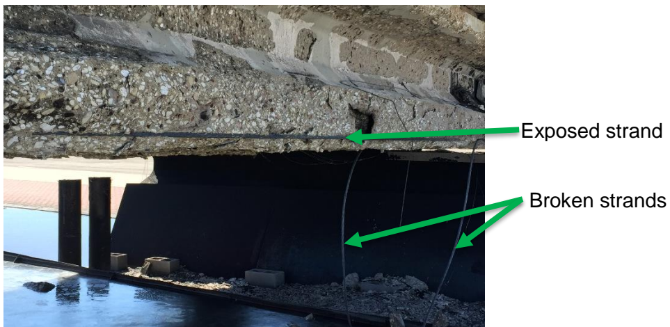
(a) Broken and exposed prestressing strands
