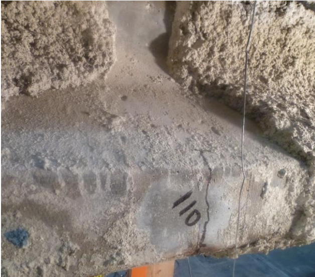
Figure 6-19 First crack on Girder-2 at 110 kips
