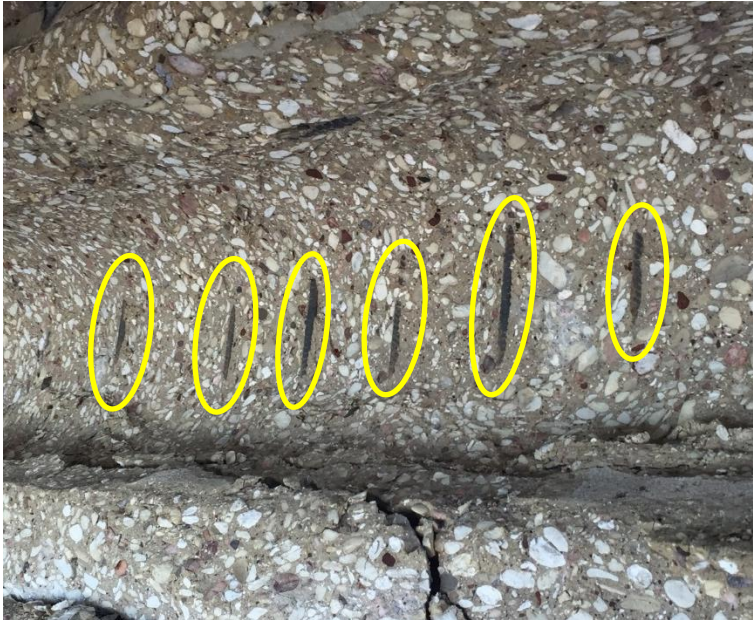
(c) Exposed shear reinforcements
