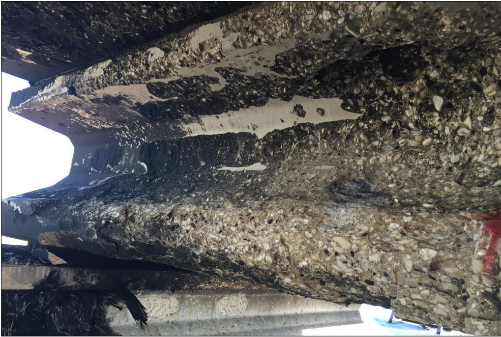
Figure 5-36 Spalling of concrete on Girder-2.
