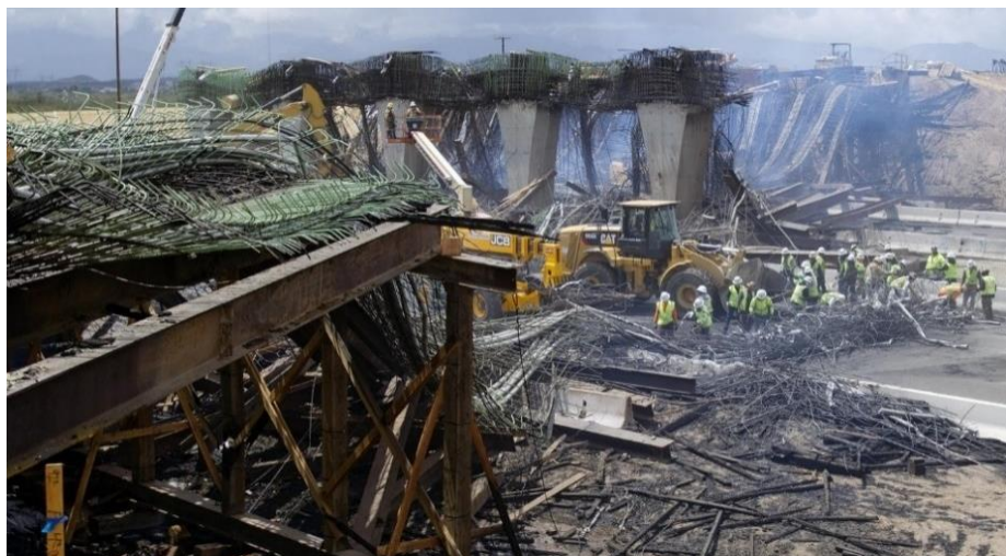
Figure 2-4 The collapse of the under-construction Rancho Road Bridge due to accidental fire (Vives et al. 2014)
