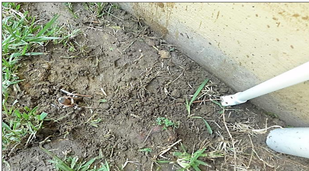
Figure 3-54 The bare copper wire is connected to the copper rod with the help of bronze clamp rod and the grounding operation is complete for the Weathering Box.
