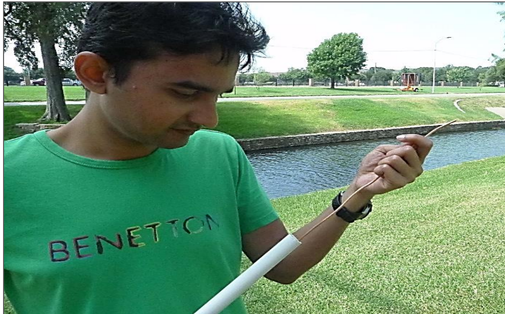
Figure 3-53 The bare copper wire is inserted into the PVC Pipe to prevent it from corroding by being exposed to the atmosphere.
