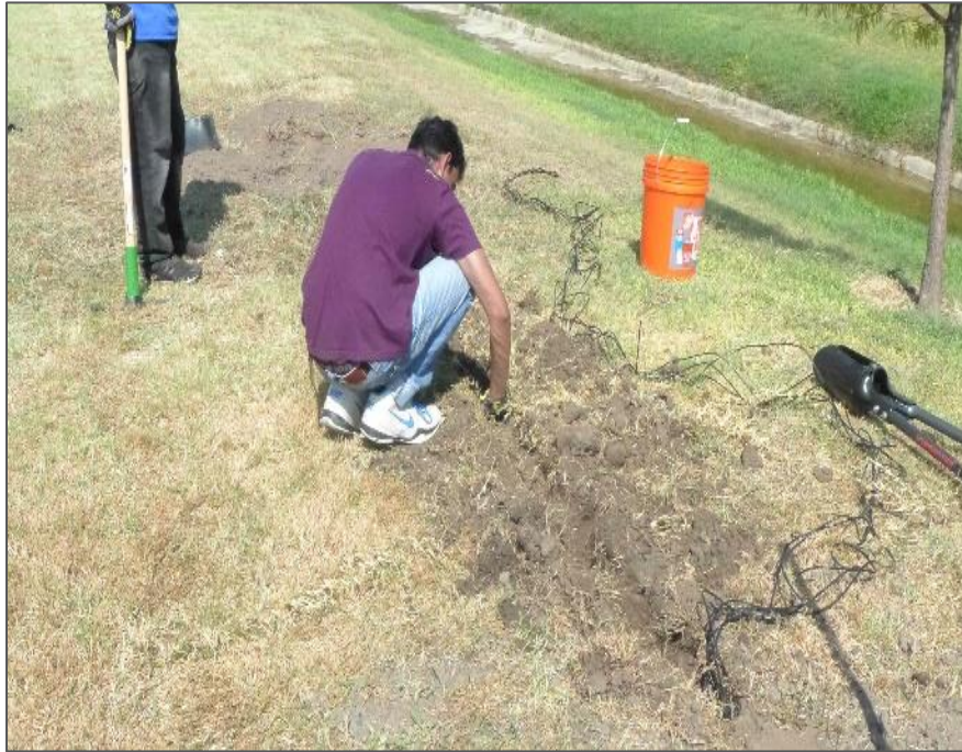
Figure 3-42 A trench of length 5 m is excavated for the irrigation wires running through to connect to the Valve Box
