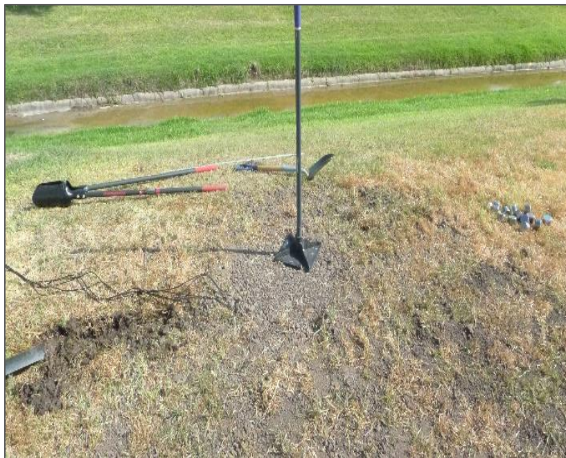
Figure 3-41 All the TDT sensors are installed and the ground surface is compacted and levelled
