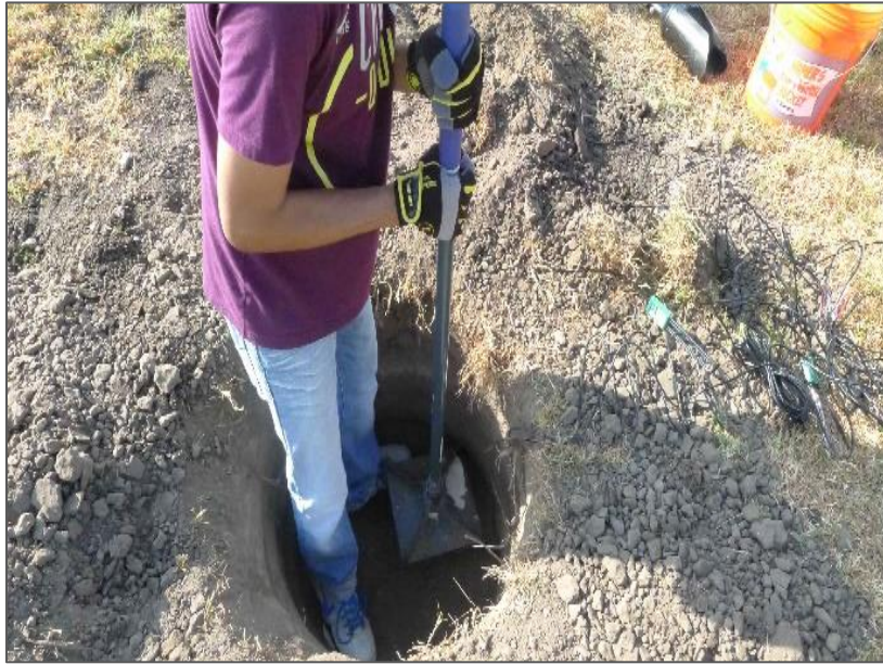
Figure 3-40 Backfill excavated soil is filled till the next depth layer and compacted with the help of tamper
