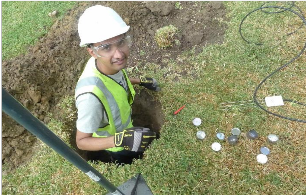
Figure 3-46 The excavated soil is leveled and compacted. Soil samples are collected at the bottom level.
