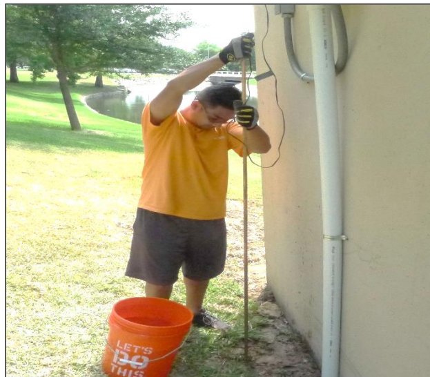
Figure 3-52 Copper Ground Rod of 5/8 inch in diameter and 8 feet long in diameter is pushed into the soil after wetting the soil
