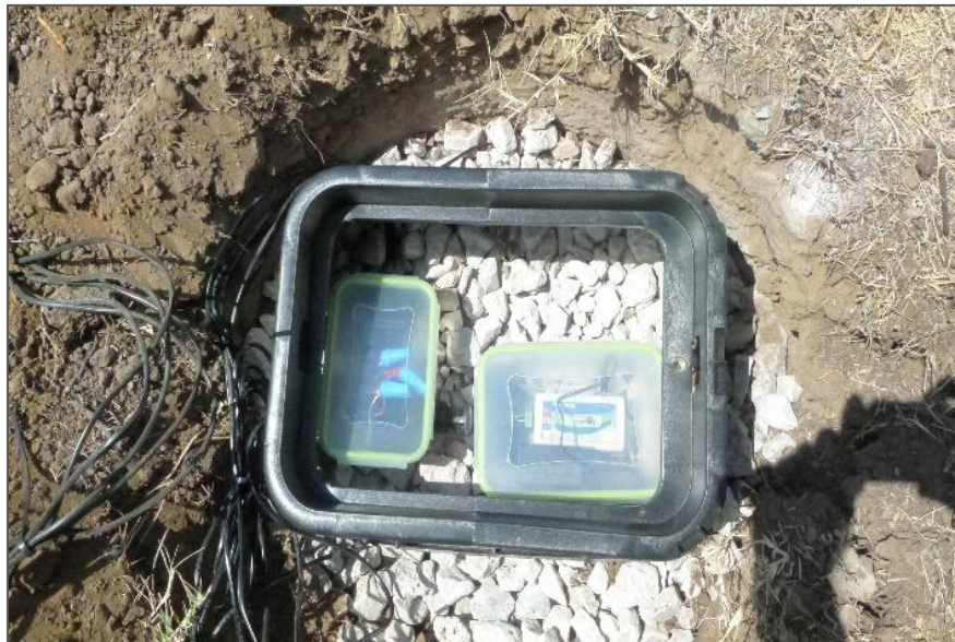
Figure 3-43 The second hole is filled with gravel and the water tight box is installed within the Valve Box with wire connection at CELB Site Location
