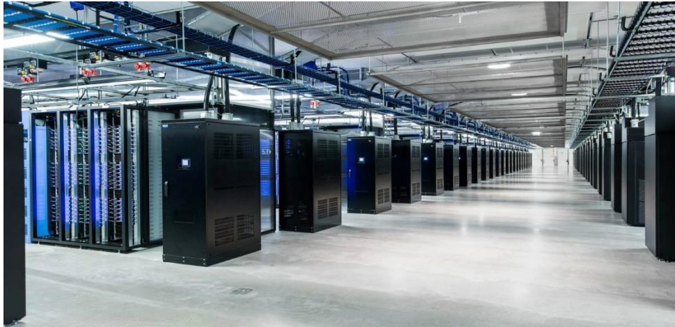
Figure 1-1 Typical interior floor space of a large data center
