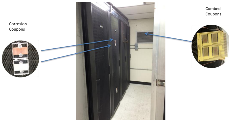
Figure 4-14: Corrosion Classification Coupon (CCC)
