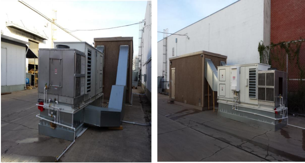
Figure 4-12: Research Modular Data Center
