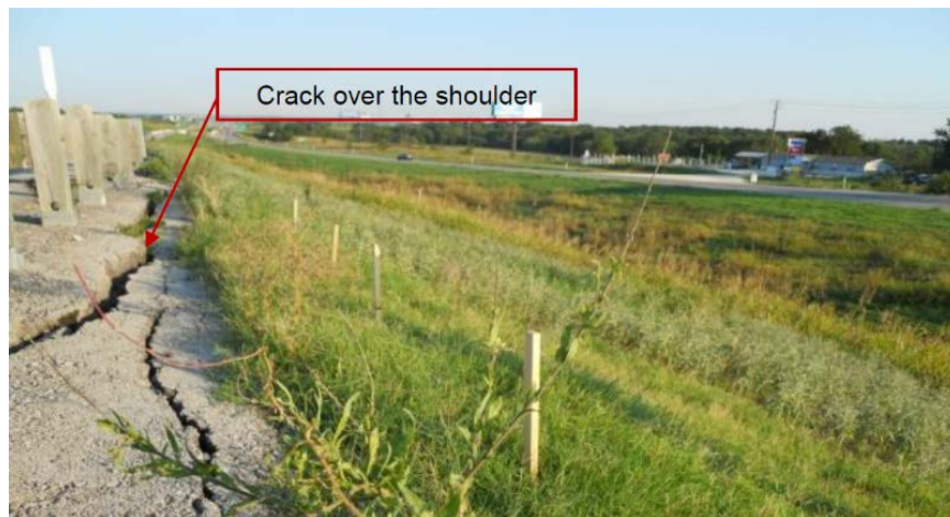
Figure 2-19 Cracks observed at the crest of the slope at US 287, Midlothian (Sadik, 2013)
