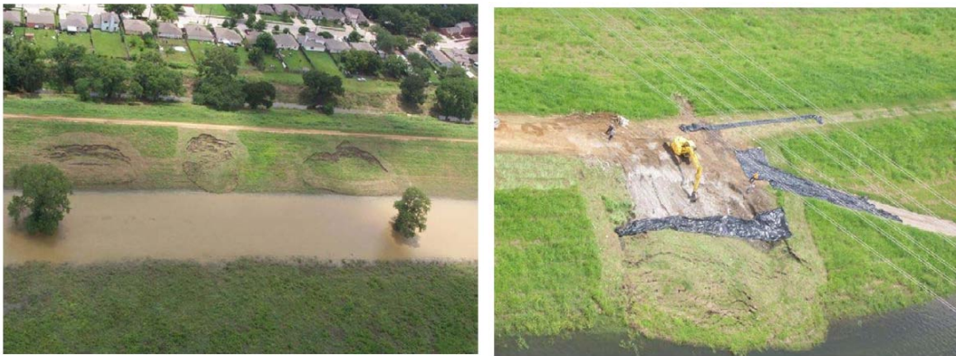
Figure 2-2 Failure occurred in Dallas Floodway Levee (Gamez and Stark, 2014)
