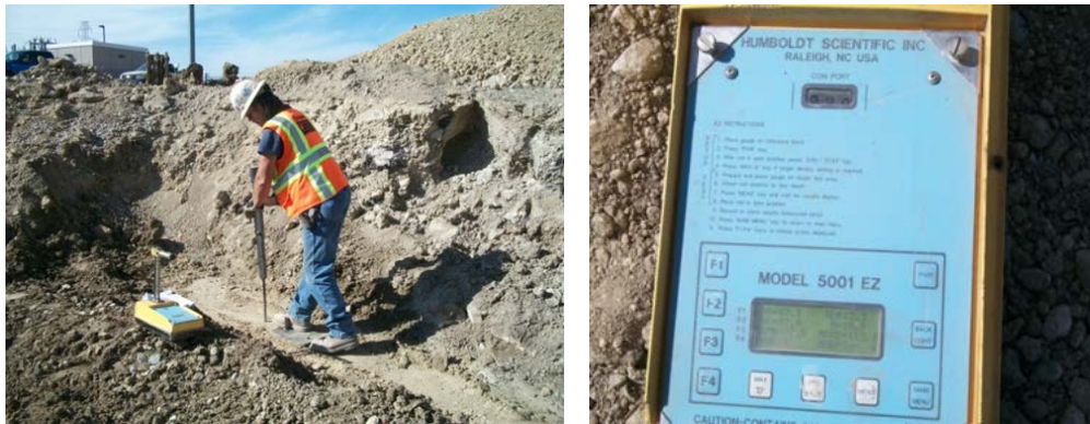
Figure 4-14 Measurement of density, compaction level, and water content of the compacted soil by using nuclear densometer
