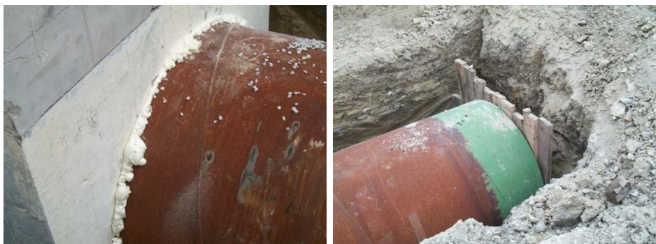
Figure 4-8 Capping and sealing the end of the pipes to prevent the flow of water or CLSM inside the pipes
