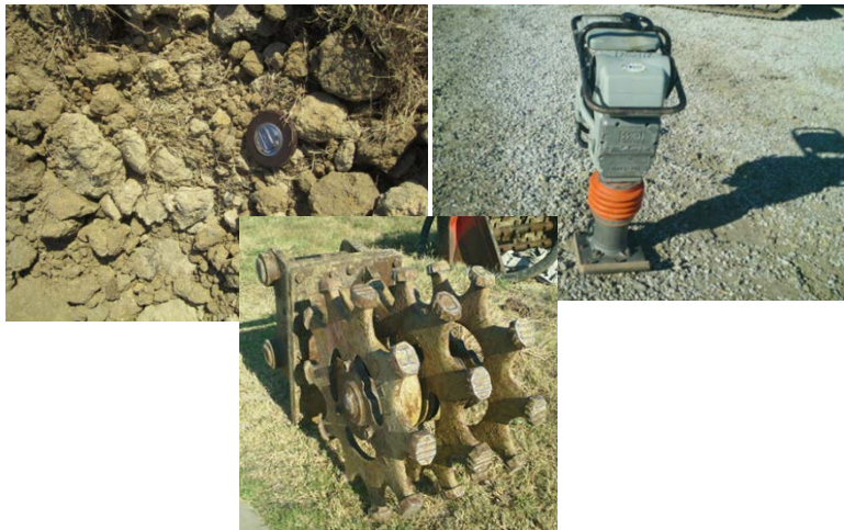
Figure 4-16 Ordinary (native) soil was compacted as backfill material with the jumping compaction and sheep feet compactor
