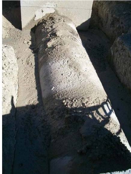
Figure 4-15 CLSM was cast for the second and third pipes up to 70% of their outside diameter
