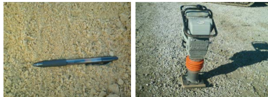
Figure 4-12 Select fill was compacted by jumping jack compactor for the first pipe
