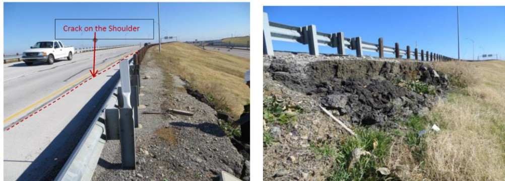
Figure 3-9 Slope failure photos at SH 183
