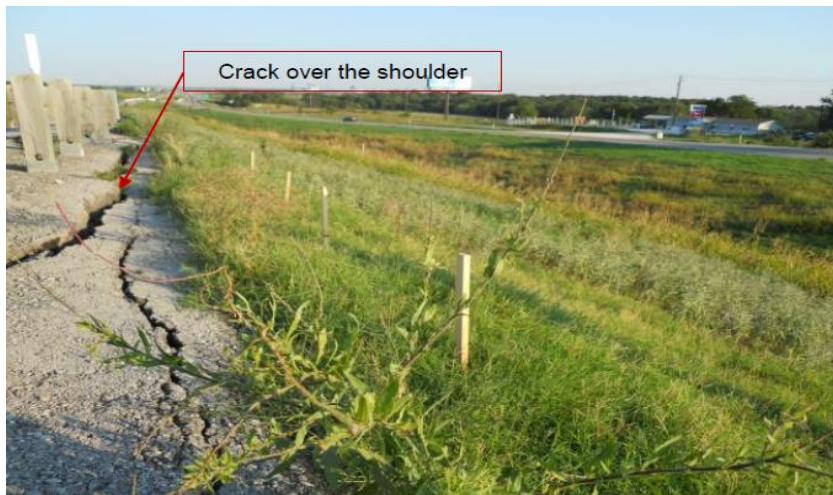
Figure 2-17 Observed cracks at US 287 slope along the crest (Khan, 2013)
