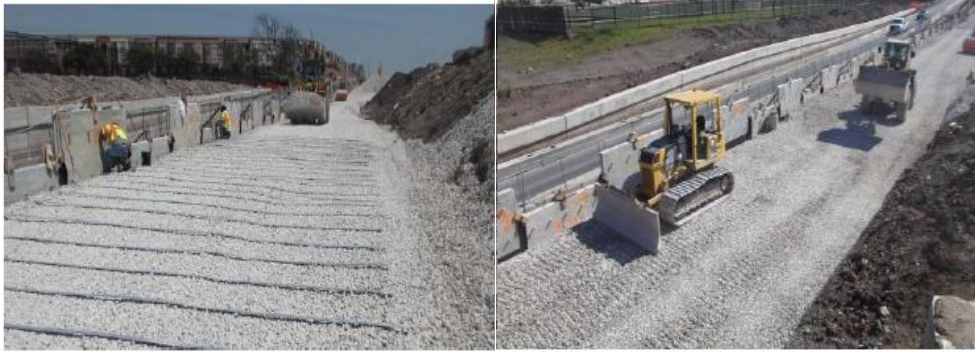
Figure 2-8 Backfilling operation in wall, strip placement over after the lift and loader compacting the backfill soil.
