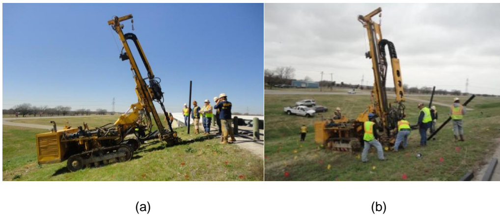
Figure 2-26 RPP instillation photo at US 287, (a) RPP instillation at Reinforced section 1, (b) RPP instillation at Reinforced section 2
