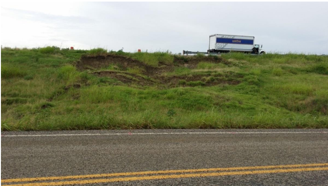
Figure 2-1 Slope Failure at US 287 north bound after heavy rainfall.
