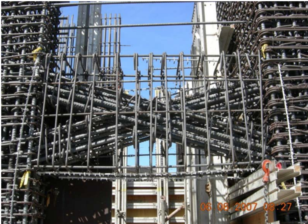
Figure 1-4 Diagonally reinforced coupling beam details with aspect ratios greater than 2.0, according to ACI 318-14 (Lequesne et al., 2010)
