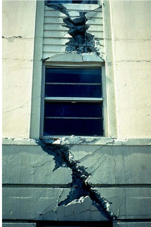
Figure 2-3 Diagonal tension failure of conventional coupling beam during Alaska Earthquake (NISEE)
