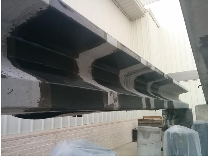
Figure 6-12 – FRP debonding at maximum loading GF1
