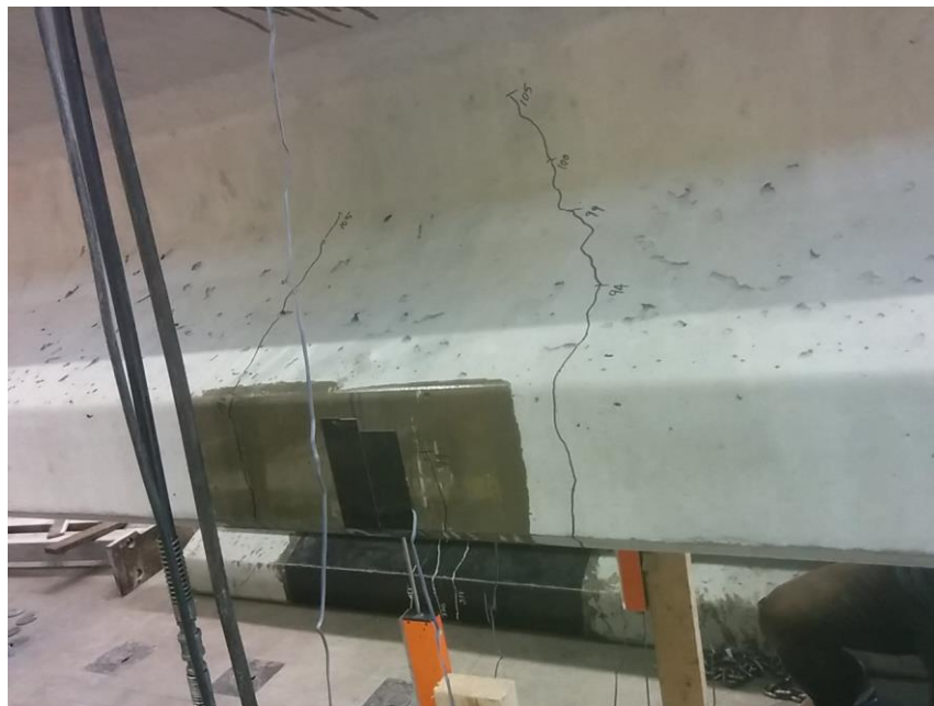
Figure 6-3 - Observed cracks due to loading GC
