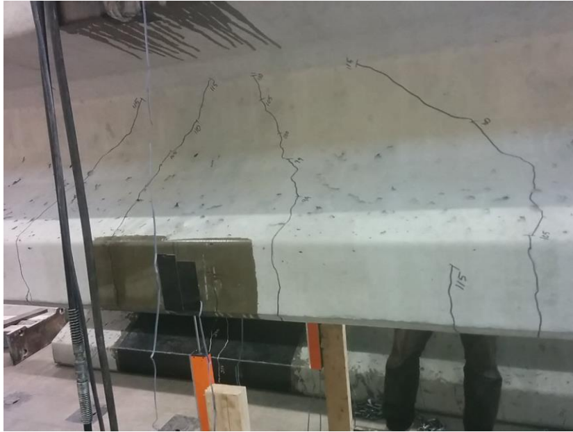
Figure 6-6 -Observed cracks due to loading GC
