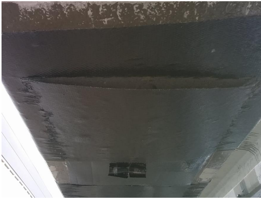
Figure 6-13 – FRP Debonding at Maximum Loading GF1
