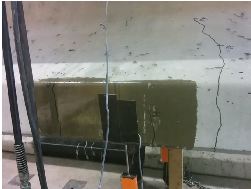
Figure 6-2 – Observed cracks due to loading GC
