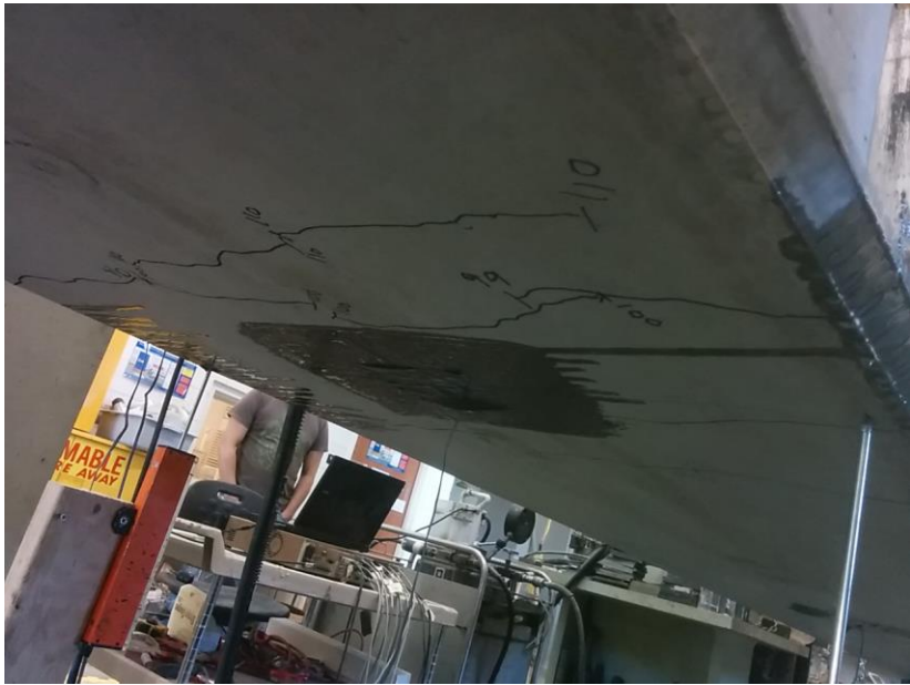
Figure 6-5 - Observed cracks due to loading GC
