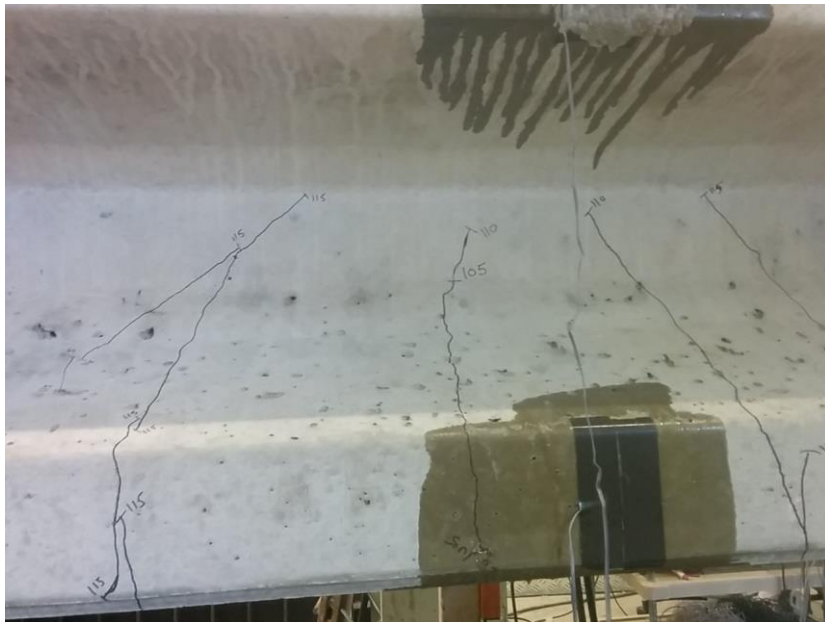
Figure 6-7 - Observed cracks due to loading GC
