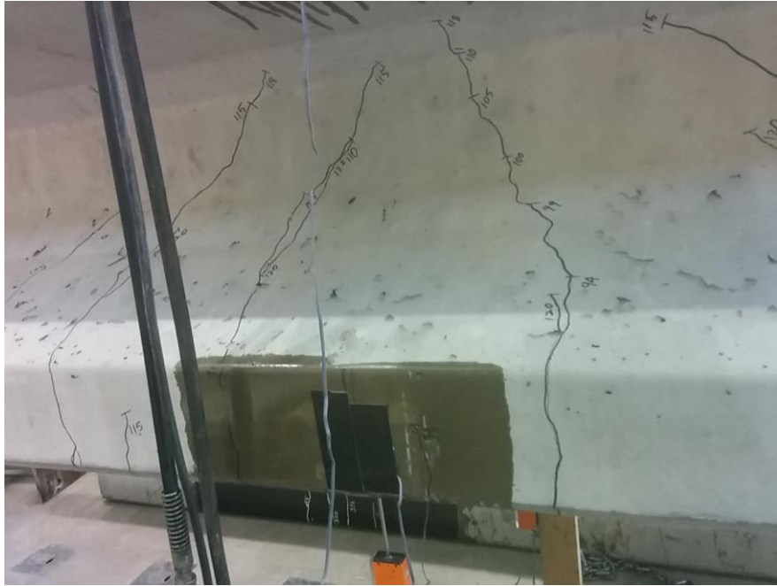
Figure 6-8 - Observed cracks due to loading GC
