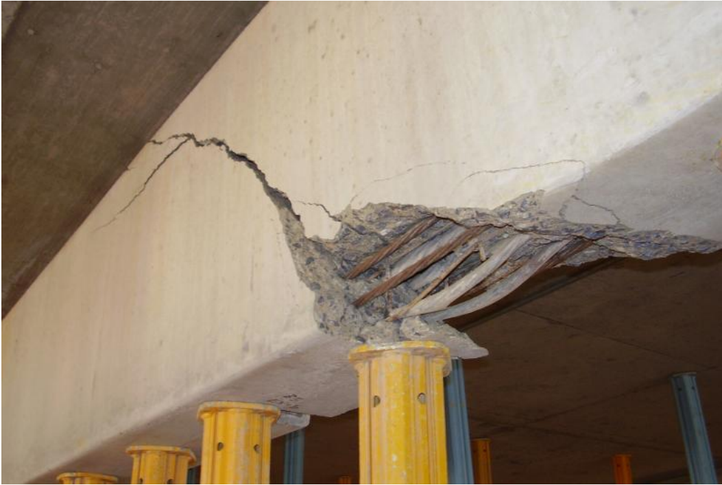
Figure 1-3 Failed post tensioned beam due to snow over load
