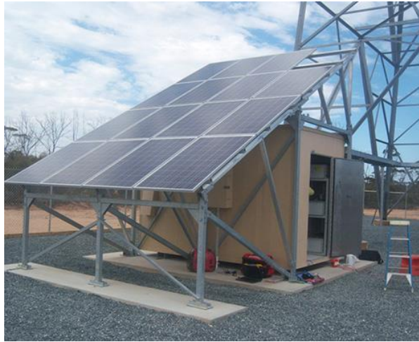
Figure 1.1 Example of PV telecomm shelter
