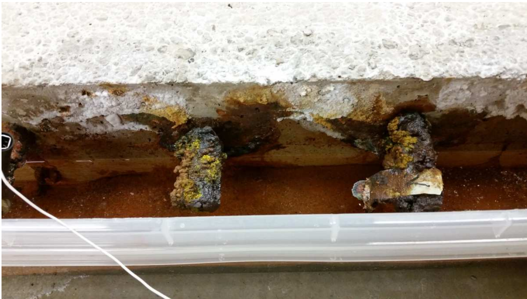
Figure 5-33 The corroded state of the two rebars in the middle after 30 days
